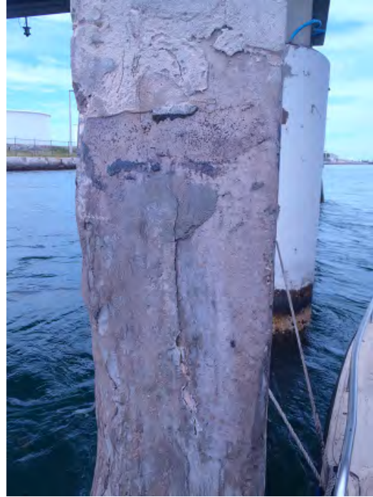
Photo No. 15: East Face of Pile 6, with vertical cracks visible in shotcrete repair.
