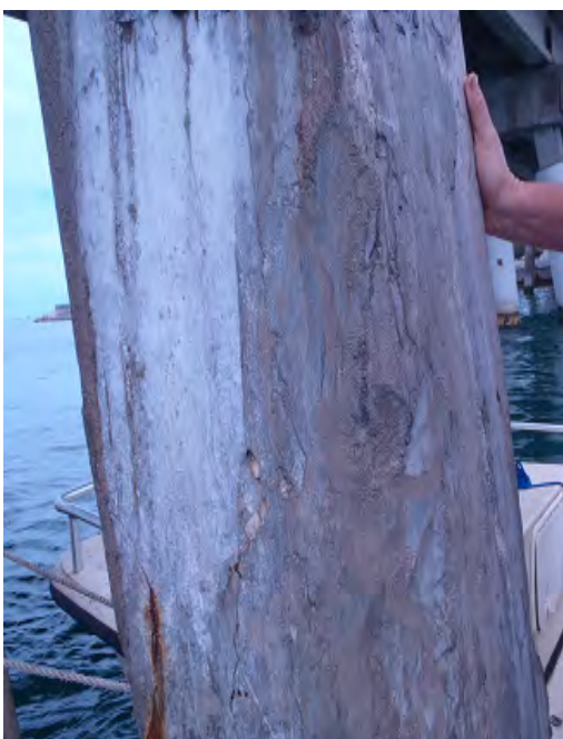
Photo No. 20: Upper portion of South Face of Pile 6, with vertical cracks visible in shotcrete repair and rust stains bleeding through.
