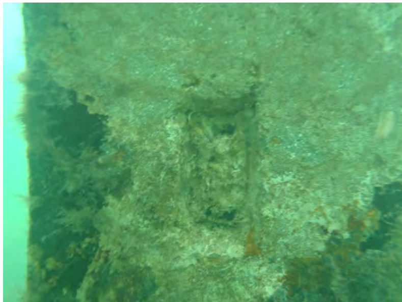
Photo No. 23: Close-up view of the West Face of Pile 5, with the depressed area visible.
