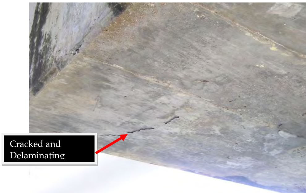
Photo No. 47: Delaminating concrete on underside, or soffit, of Pile Cap 14-15.
