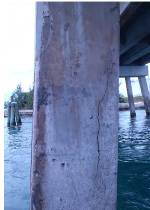
Photo No. 17: South Face of Pile 6, with vertical cracks visible in shotcrete repair. Vertical cracks extend beyond the limits of the shotcrete repair and into the concrete pile itself.
