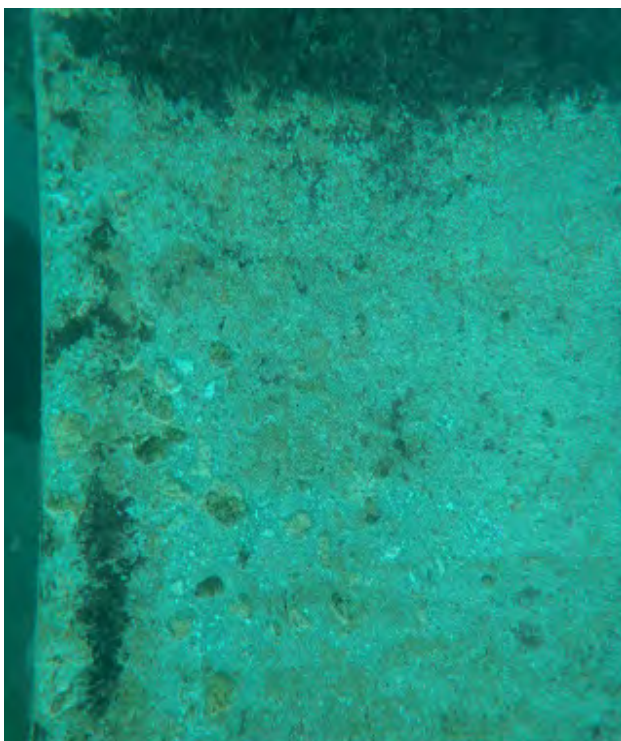
Photo No. 25: Close-up view of the East Face of Pile 9, with minor pitting visible.
