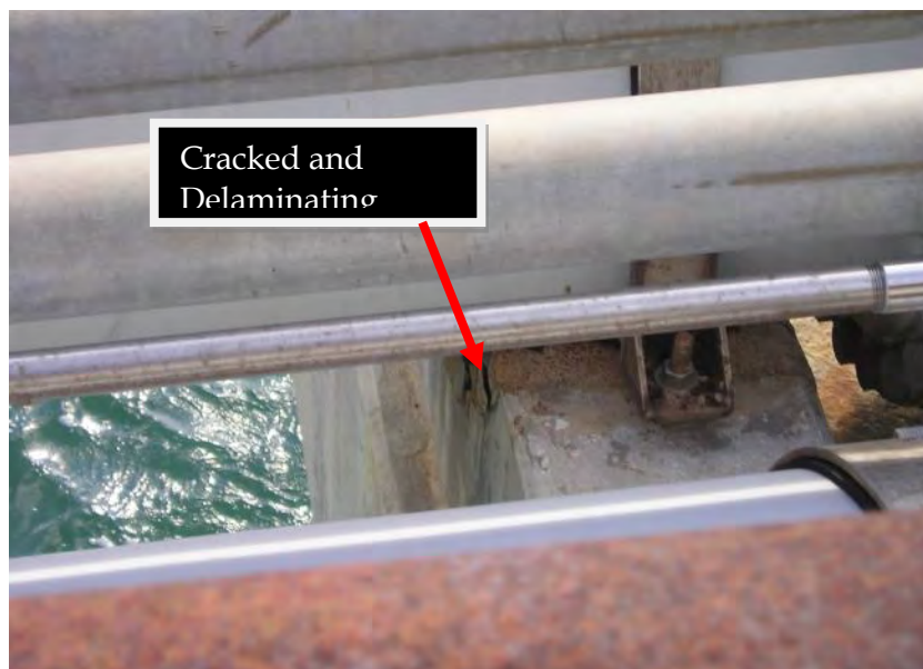
Photo No. 38: Cracked and delaminating concrete visible on north side of pipe support on Pile Cap 3-4.
