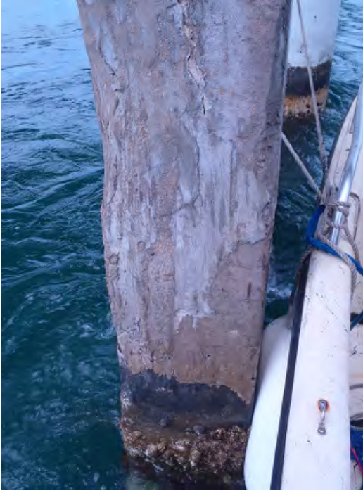
Photo No. 14: Above water view of the East Face of Pile 6, with vertical cracks visible in shotcrete repair.
