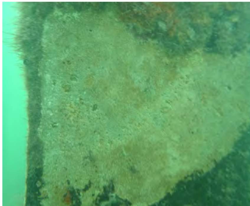
Photo No. 11: Close-up view of West Face of Pile 7, with minor pitting visible.
