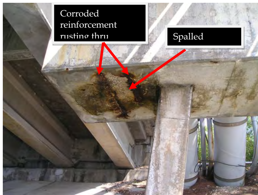
Photo No. 34: View of Pile Cap 12-13 and Pile 13, with rust stains from corroded reinforcement bleeding through pile cap soffit and spalled concrete pile cap soffit.
