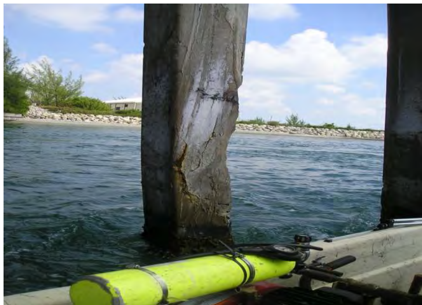
Photo No. 41: Close-up view of damaged Pile 6, with cracked and delaminated shotcrete repair visible.
