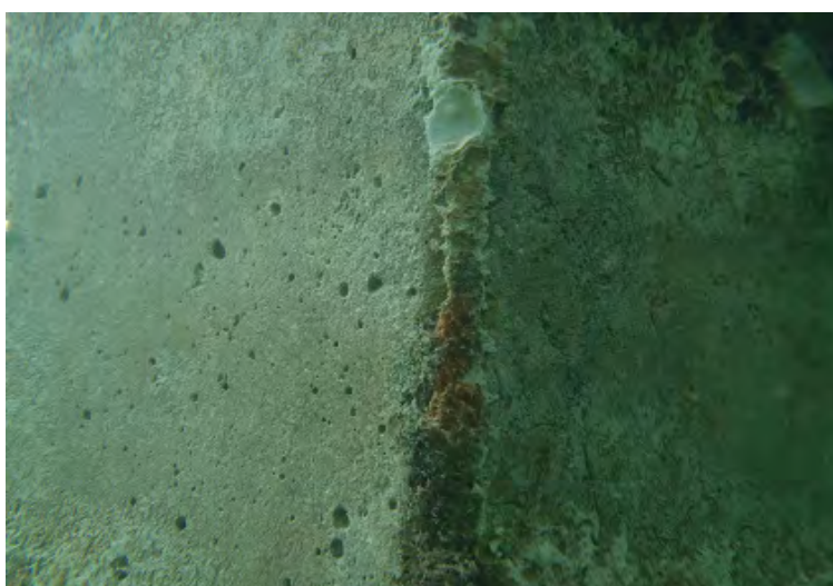
Photo No. 5: Close-up view of Northwest Corner of Pile 2, random pitting visible.
