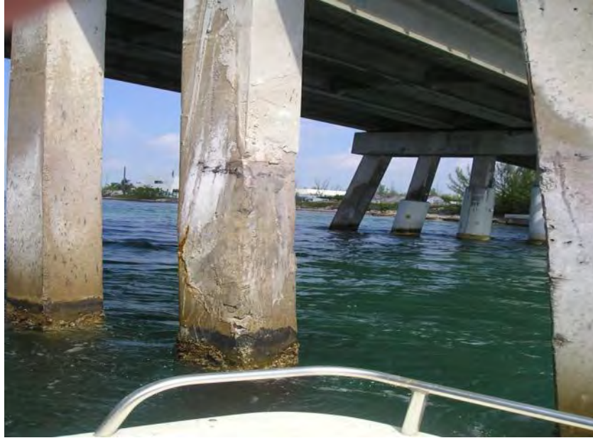
Photo No. 40: Damaged Pile 6, with Pile 7 to the left and Pile 5 to the right.
