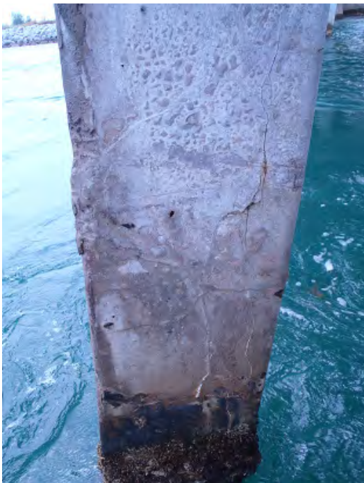
Photo No. 16: Above water view of the North Face of Pile 6, with cracks visible in shotcrete repair.
