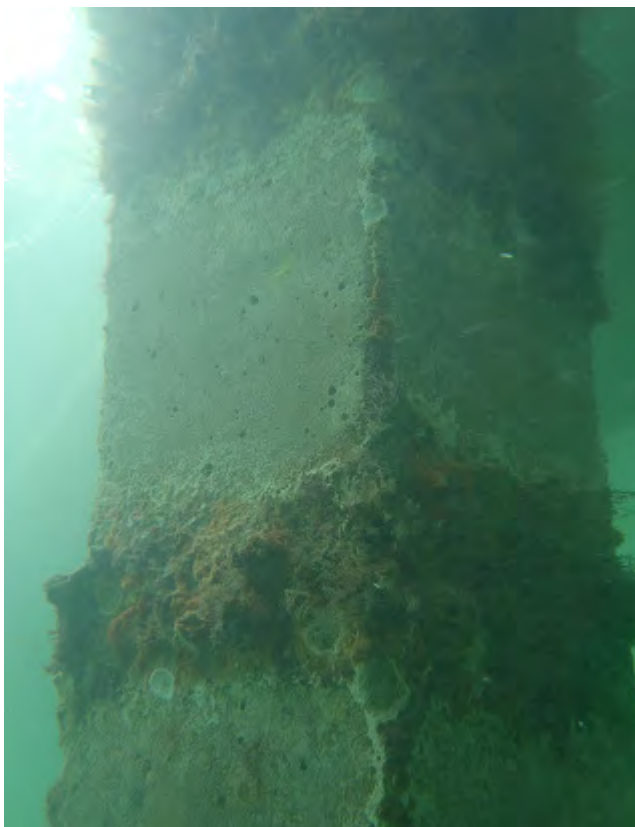
Photo No. 4: Northwest Corner of Pile 2, random pitting visible.
