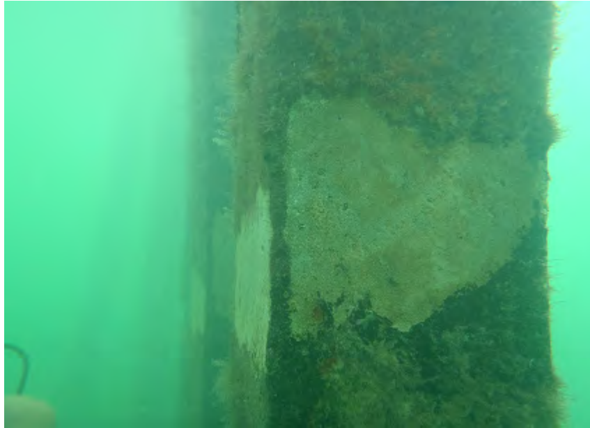
Photo No. 10: West Face of Pile 7, with minor pitting visible.
