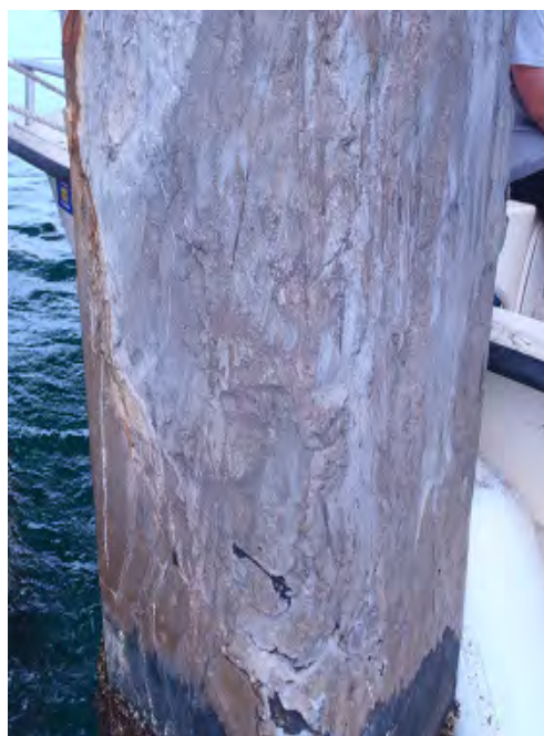
Photo No. 21: Lower portion of South Face of Pile 6, with vertical cracks visible in shotcrete repair and rust stains bleeding through.
