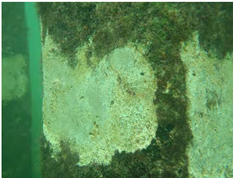
Photo No. 13: Close-up view of Southeast Corner of Pile 6, with minor pitting visible.
