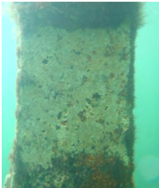
Photo No. 9: Close-up view of North Face of Pile 3, with marine growth removed and pitting visible.
