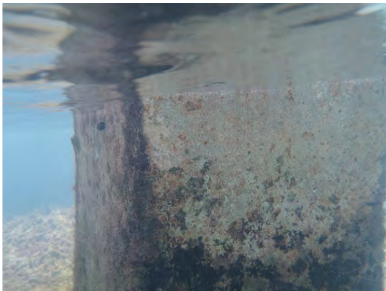
Photo No. 3: West Face of Pile 12, with no apparent pitting visible.
