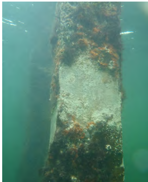
Photo No. 7: East Face of Pile 4, with marine growth removed and minor pitting visible.
