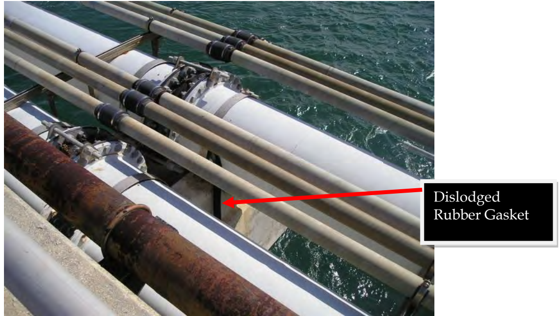
Photo No. 44: Dislodged rubber gasket at pipe clamp at Pile Cap 10-11.
