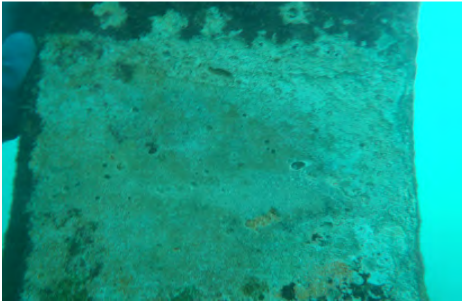
Photo No. 26: Close-up view of the South Face of Pile 8, with minor pitting visible.
