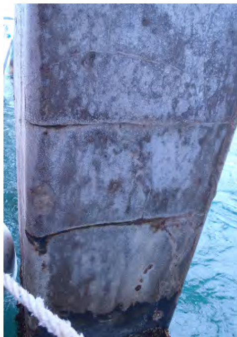
Photo No. 19: West Face of Pile 6, with horizontal cracks visible, with rust stains bleeding through.
