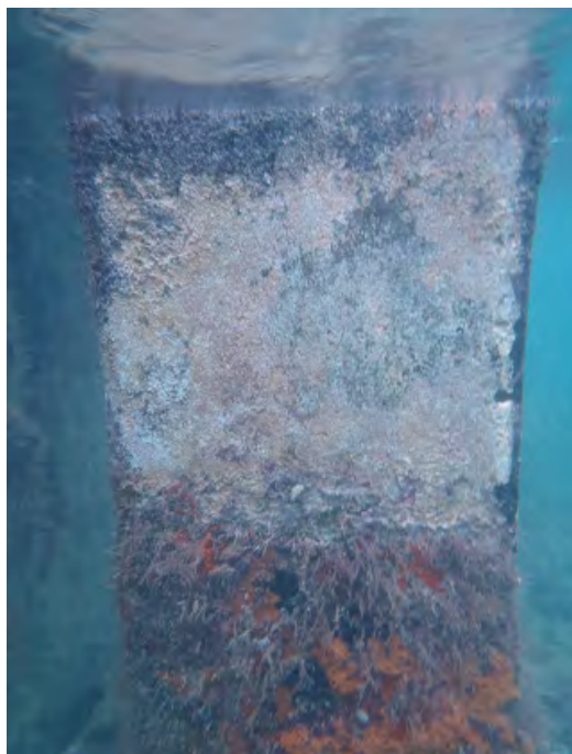
Photo No. 29: Close-up view of East Face of Pile 15, with minimal pitting evident.
