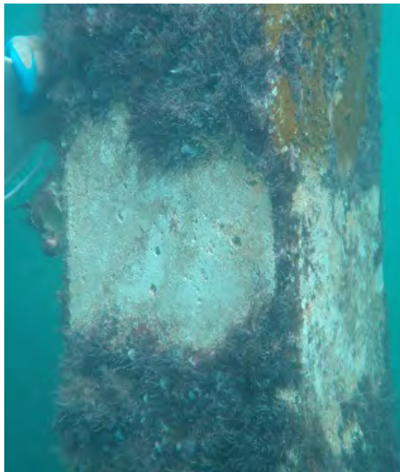
Photo No. 27: View of South Face of Pile 11, with minor pitting visible.
