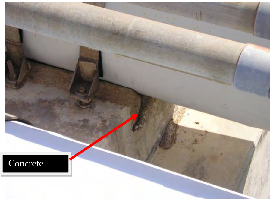
Photo No. 46: Concrete spall on south side of pipe support on Pile Cap 14-15.
