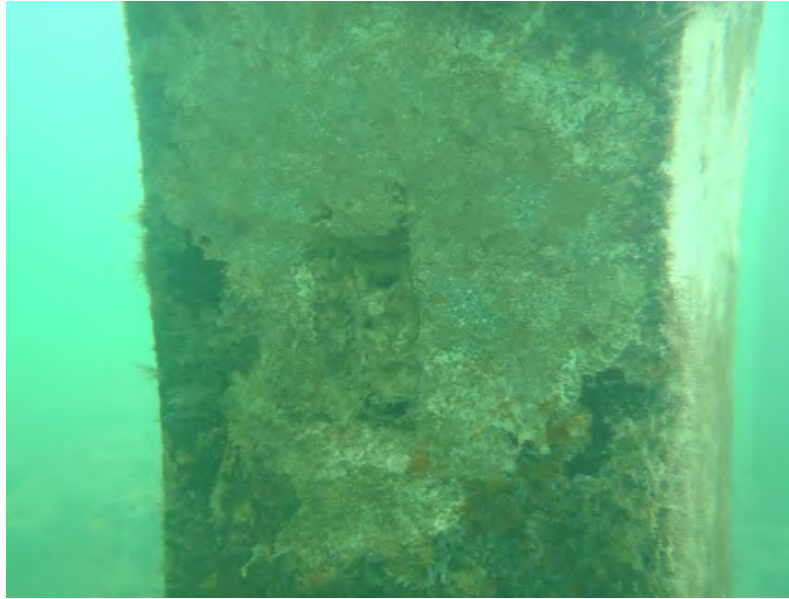
Photo No. 22: West Face of Pile 5, with the depressed area visible.
