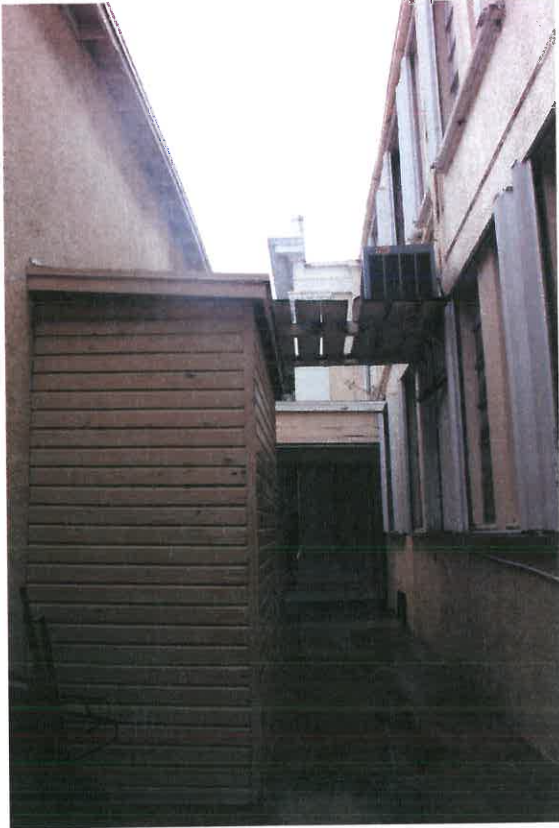
Shed and a/c overhang between Buildings A and B. Both are to be removed in Spring 2014.
