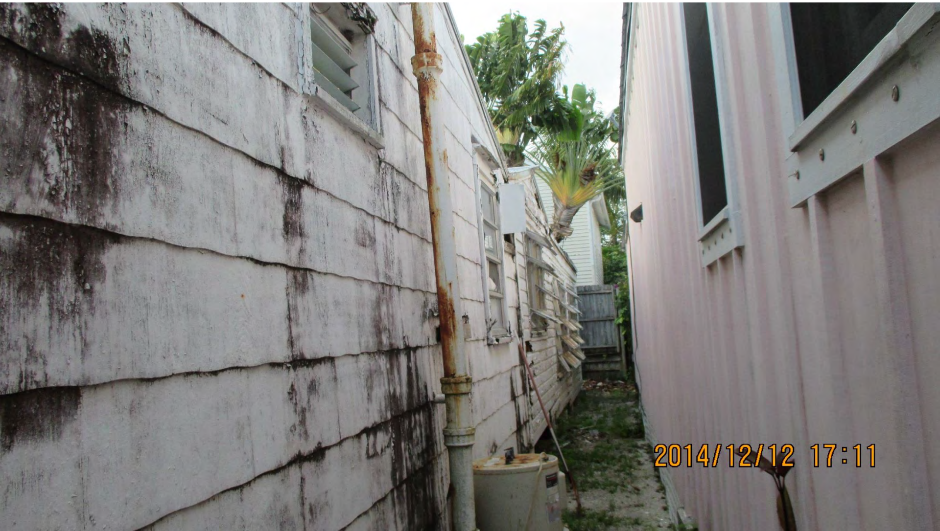
Asbestos siding on the main house and the shed roof addition. Novelty siding on the other rear additions. Note the board and batten siding on the neighboring house at 1311 Newton.
