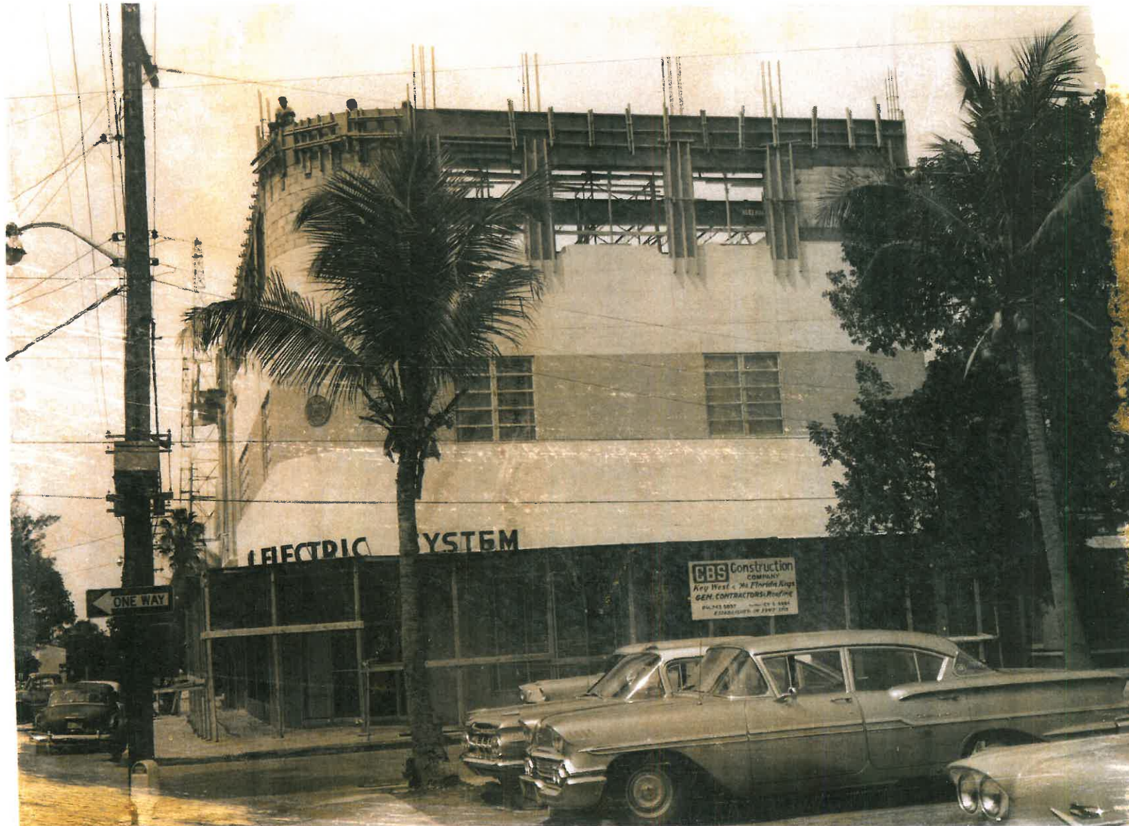
#533 Eaton Street circa 1961 when third floor was under construction. Monroe County Library
