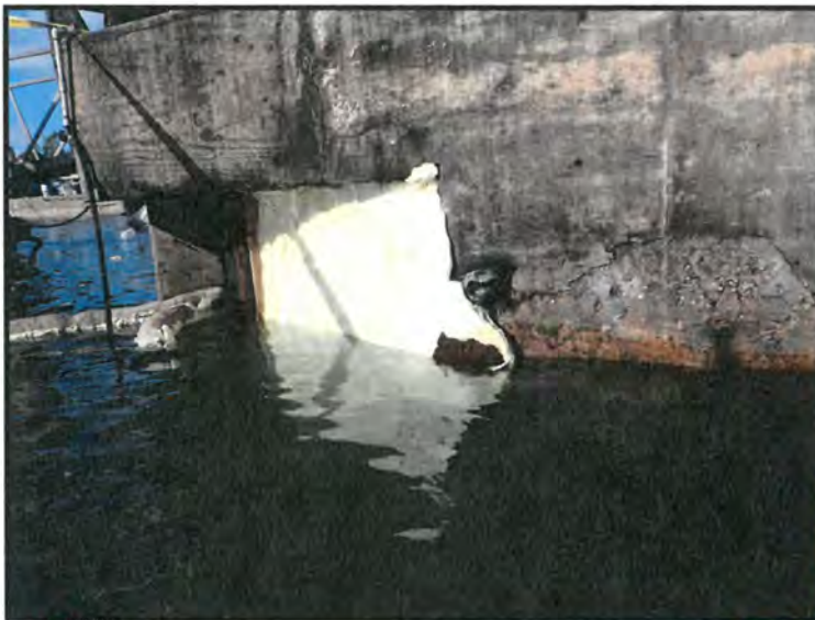
To the left is a picture of the repair of the seawall within the travel lift basin.
