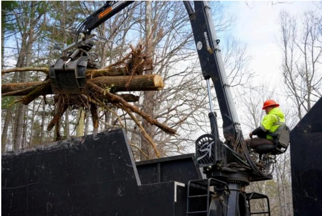
Visual reference: controlled grapple loading near storm-damaged trees using PPE and trained operators.
