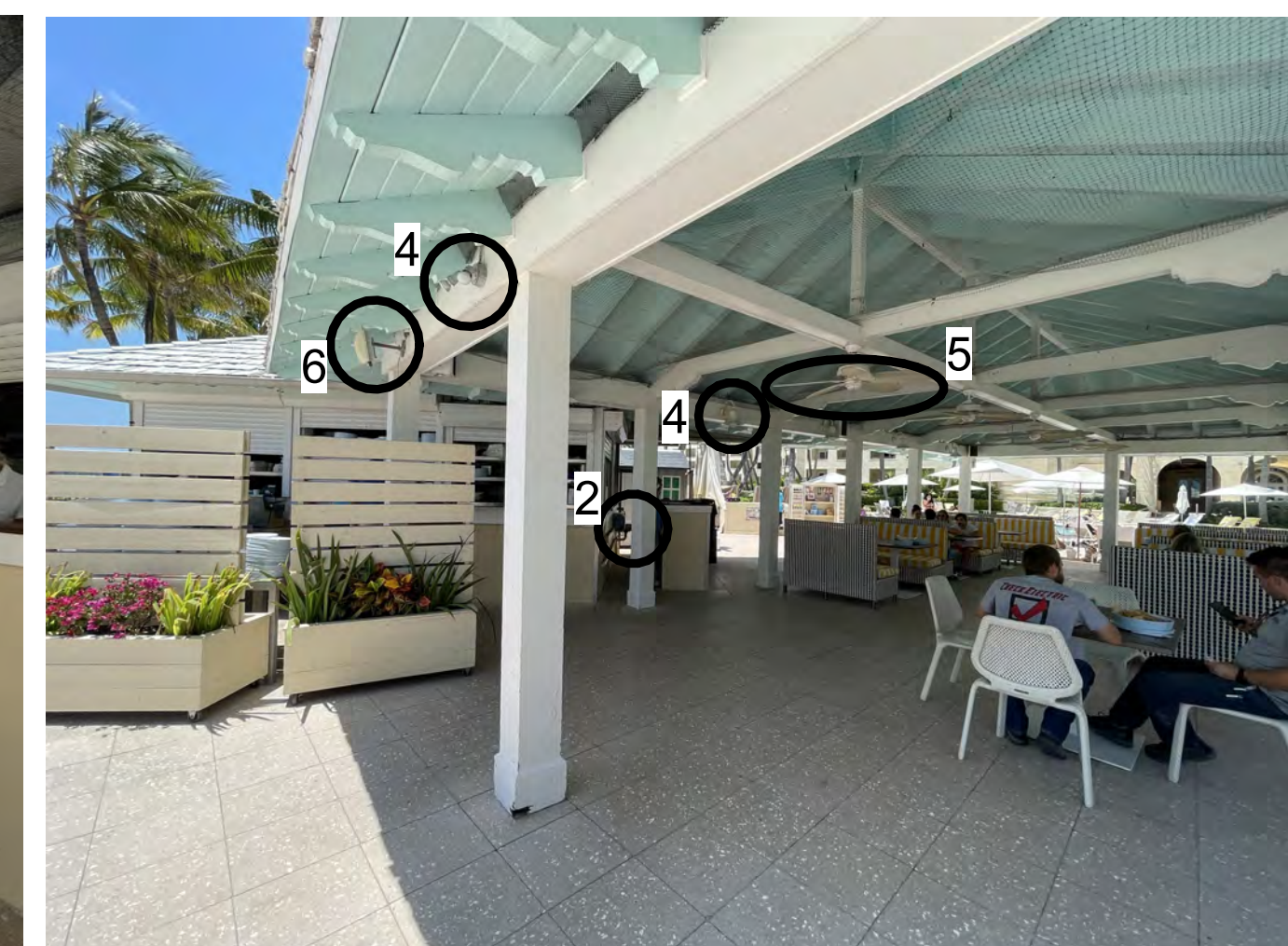
B2 REMOVE AND SALVAGE TO RETURN TO OWNER, TYPICAL THROUGHOUT SPACE 2. SINK AND ACCESSORIES 4. EXTERIOR LIGHTING 5. FANS 6. SPEAKERS
