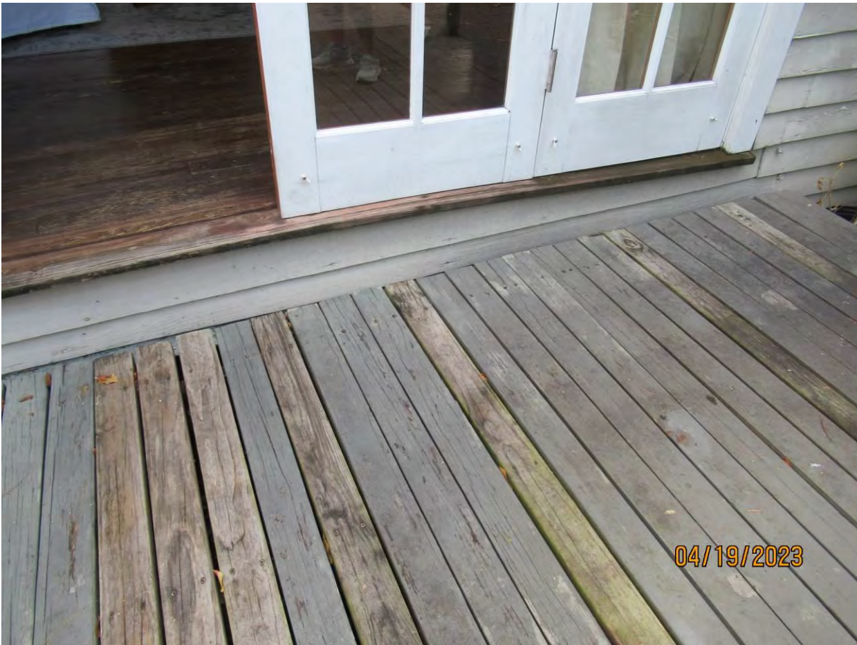
Photo showing floor raised near tree.
