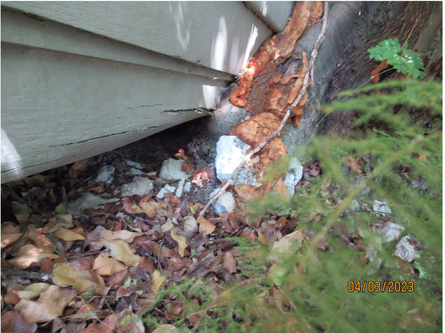
Photo showing base of tree at base of structure.
