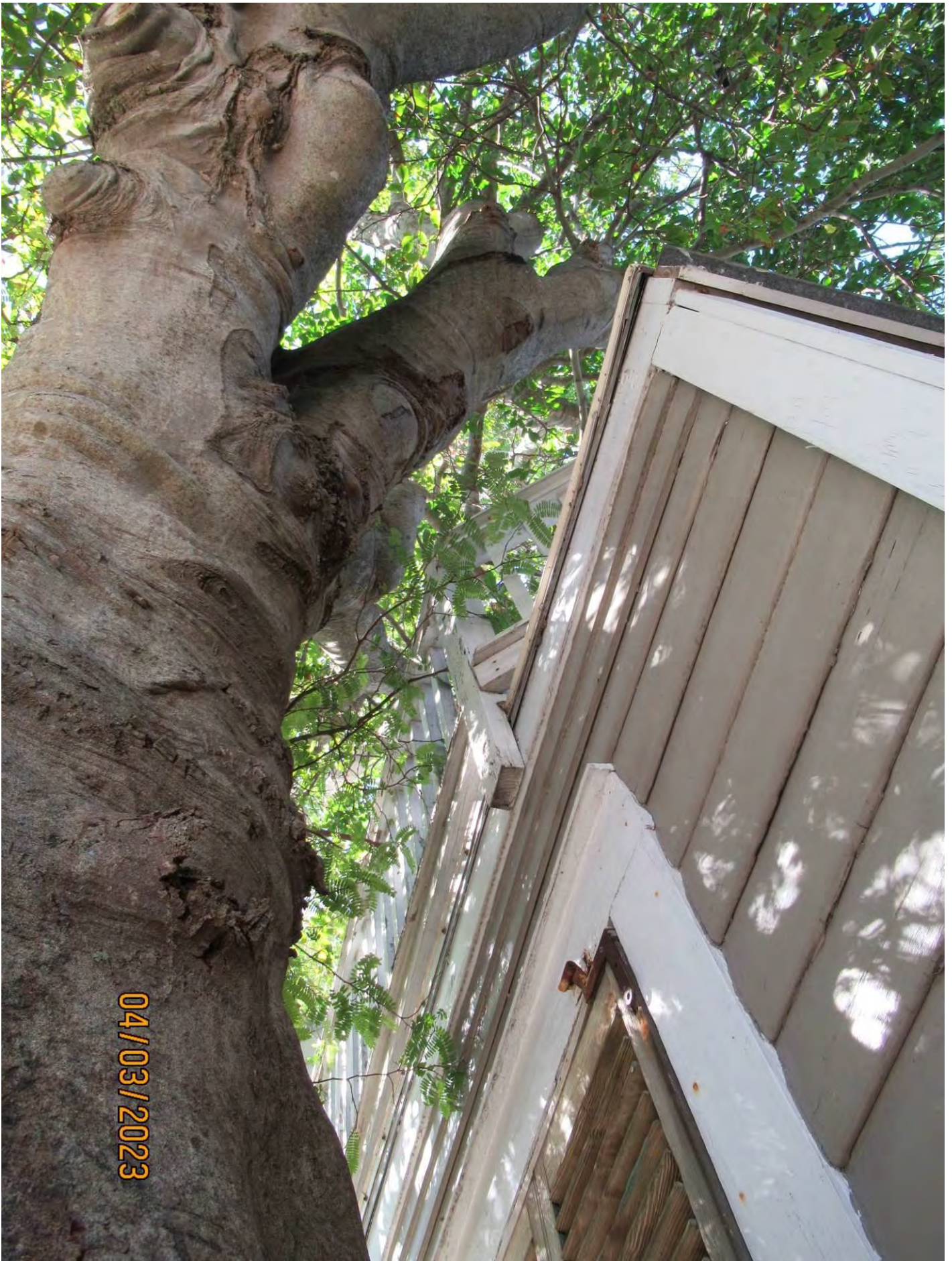
Photo showing tree trunk and canopy in relation to structure.
