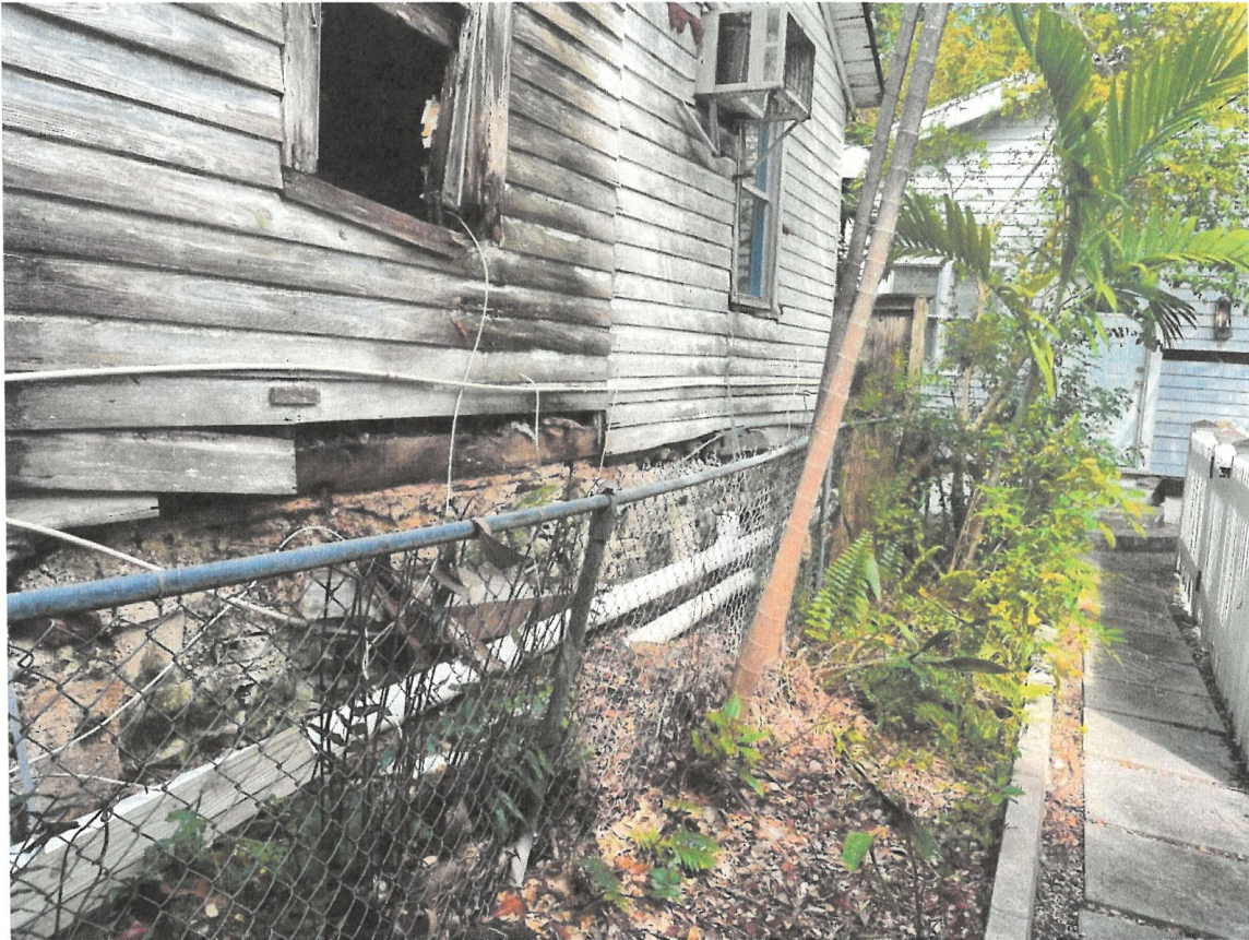
Photograph 4: Photograph of the exterior showing the damaged siding, rim beam and deteriorated foundation.
