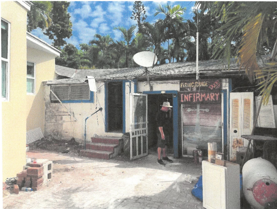
Photograph 1: View of the entrance to 703 Windsor. The asphalt shingle roof, windows and walls appear in poor condition. The structure is connected to 627 Elizabeth Street on the left and 705 Windsor on the right.
