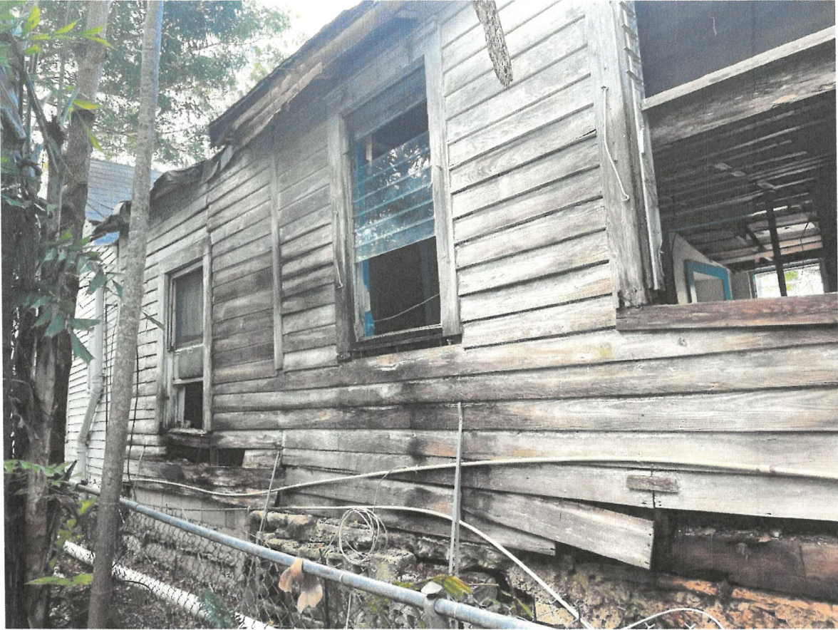
Photograph 5: Photograph of exterior showing damaged windows and rotten siding.
