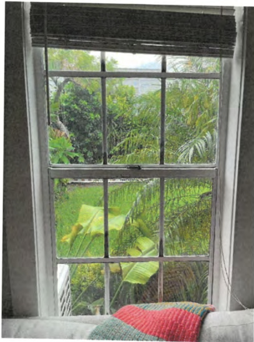
Figure 14 – Southernmost window on east side of existing residence, to be removed (interior)
