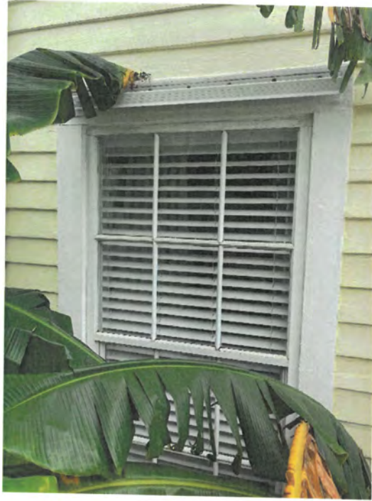
Figure 13 – 2nd window from the south on east side of existing residence, to be removed (exterior)
