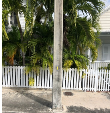
West view – utility pole obstruction
