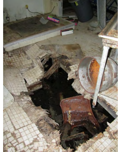
Interior view of the West Cable Hut, showing the collapsed floor. Restaurant equipment has fallen through the plywood floor into the flooded crawlspace below.
