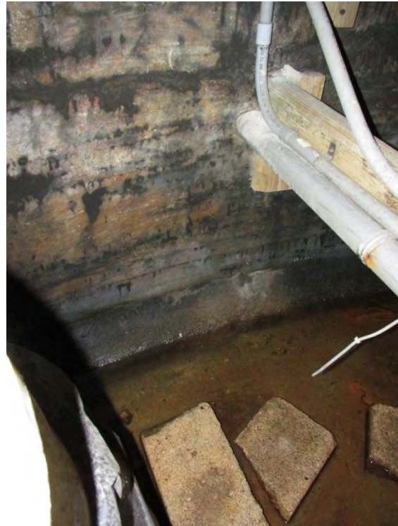
The original concrete wall and floor of the East Cable Hut can be seen in this photo. The concrete floor of the tank lies approximately 36" below grade, and is flooded with approximately 3" of water.
