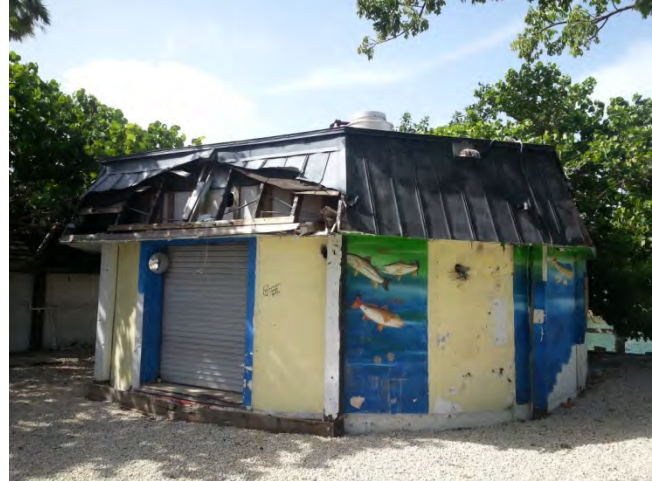
General view of the West Cable Hut. The concrete exterior walls have been covered in murals. Note the large openings cut into the walls for doors. The mansard upper roof structure has been covered with v-crimp roofing, much of which is damaged.
