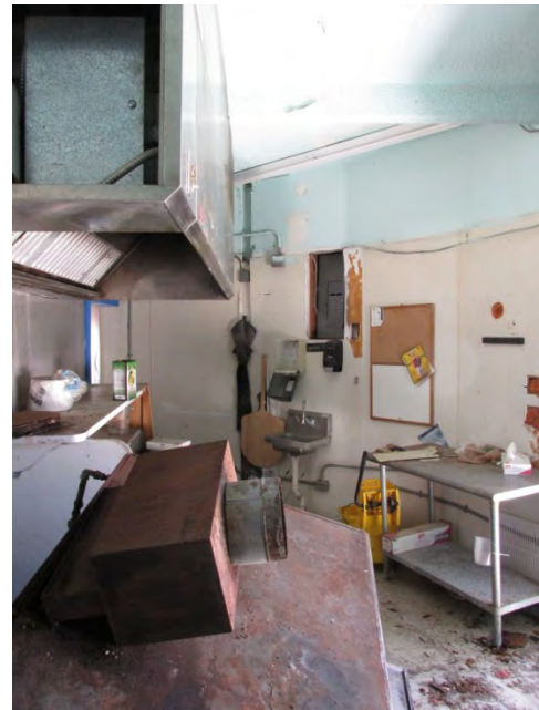
A view of the restaurant kitchen at the West Cable Hut. The pizza oven at foreground has fallen through the rotted floor. Electrical conduit can be seen running along the walls.
