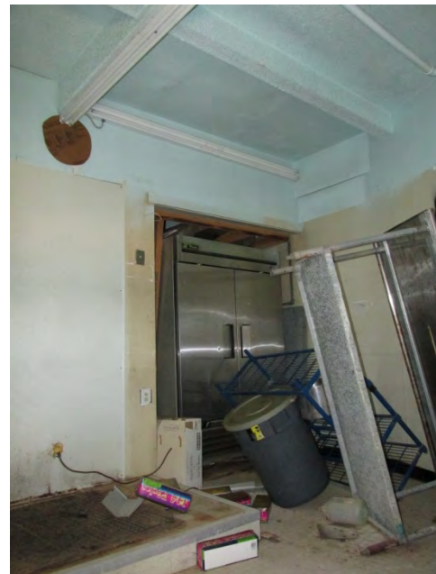
Typical interior view of the West Cable Hut, showing painted gypsum board ceilings, FRP walls, and Vinyl flooring. Note decayed restaurant equipment.
