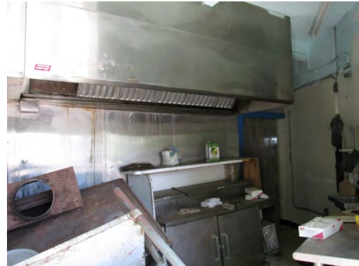
The existing hood vent at the West Cable Hut.
