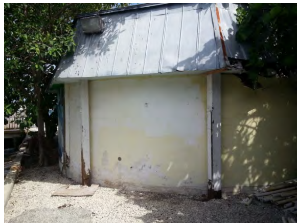
The exterior of the West Cable Hut, showing the 6" x 8" heavy timber columns ringing the tank. The columns are deteriorated at their bases, but otherwise appear in good condition.
