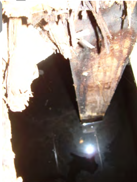
Column into water with no visible protection.
