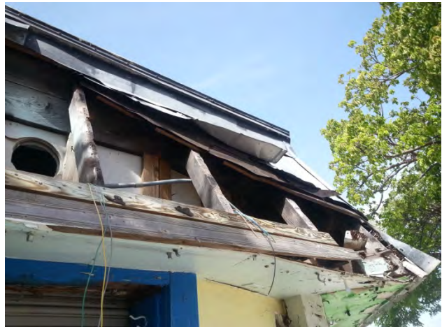
The West Cable Hut mansard roof, showing damaged v-crimp roofing. Parts of the roof framing are original, but have been heavily altered.
