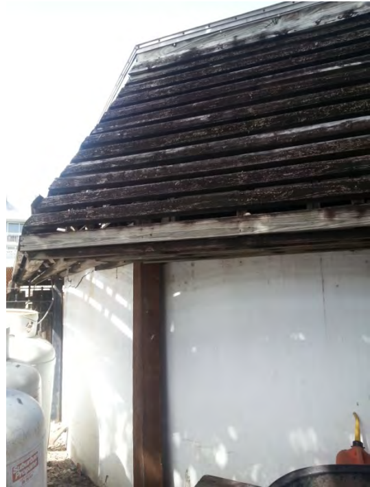
Close-up view of the roof edge of the East Cable Hut. This roof consists of 2x4's gapped 5" o.c. over a 2x wood frame.
