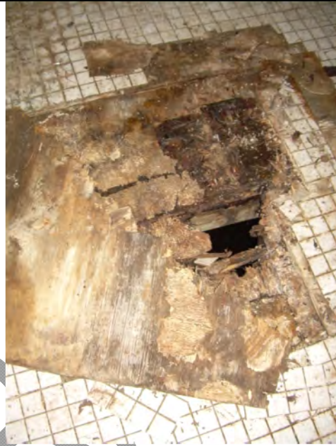
Hole in wood floor framing (water below).
