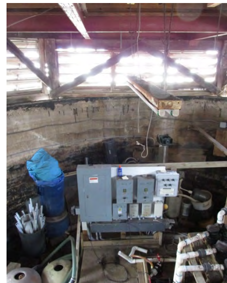
Interior view of the East Cable Hut, showing the pumps. The electrical panels are visible at center. The series of water pumps can be seen at right. At the center of the photo is a plywood floor. A hole has been excavated under this floor to access seawater from below grade.
