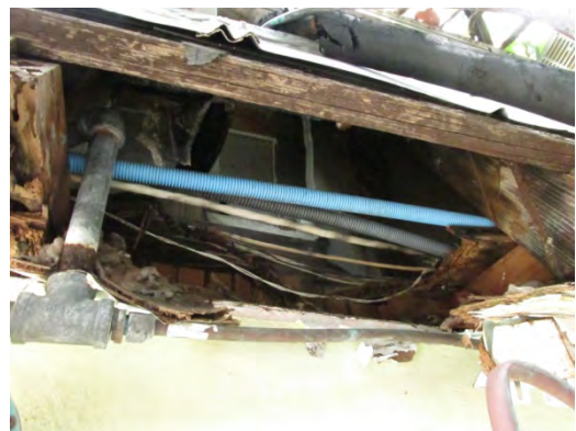
A view of the existing exterior soffit at the West Cable Hut. Several utilities are exposed, including wiring in flexible conduit, gas lines, romex conduit, and what appears to be low voltage wire.
