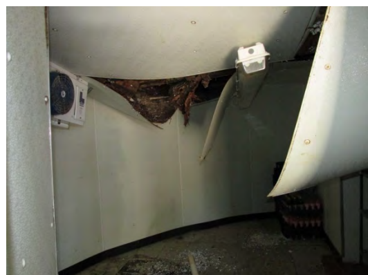
A view of the walk-in refrigerator at the West Cable Hut. The ceiling has collapsed due to leakage.
