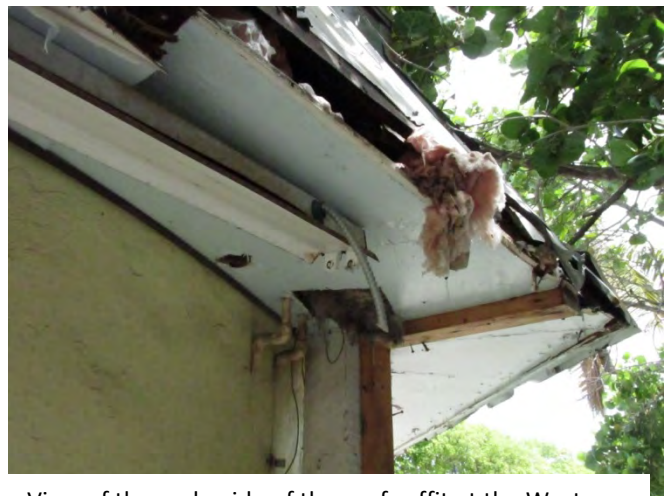
View of the underside of the roof soffit at the West Cable Hut. While the mansard structure is likely historic, it has been heavily altered with the addition of insulation, plywood soffits, wiring, and lighting.
