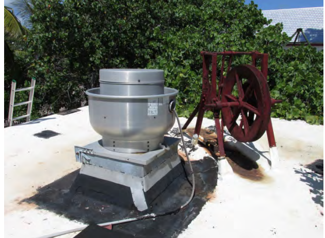
General view of the West Cable Hut roof. The Ansul hood vent is at left and the historic cable winch is at right.
