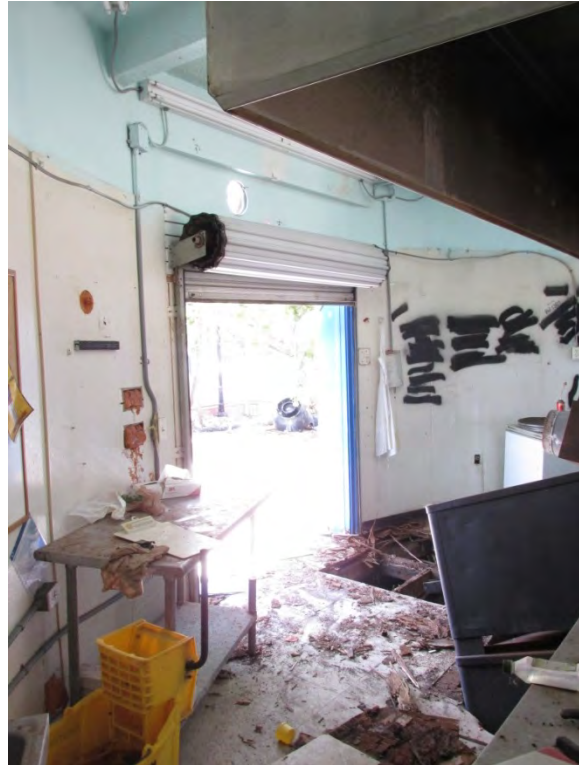
The interior of the West Cable Hut. The collapsed wood framed floor can be seen in the background. The dark object at right is a large pizza oven which has fallen through the floor into the flooded crawlspace below.
