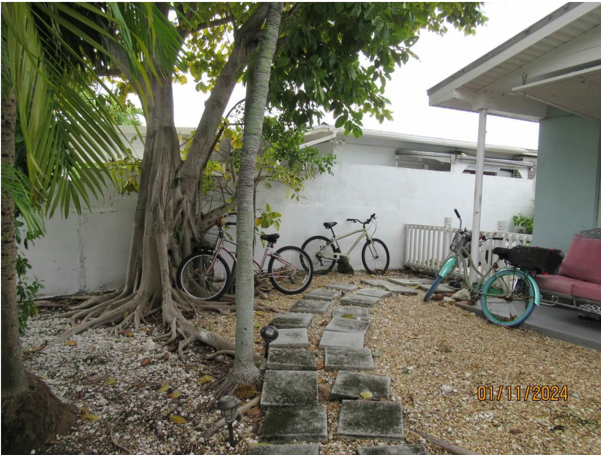
Photo of tree trunks and roots and their relationship to primary structure.
