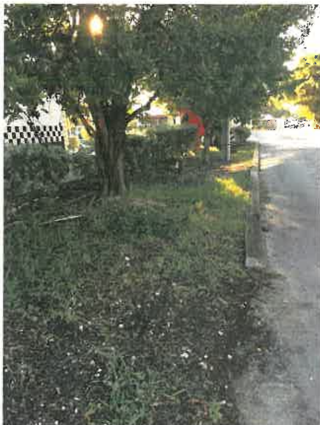
Existing Curbing on 7 th Street Side to Be Replaced with 8" Retaining Curb for Drainage Swale.
