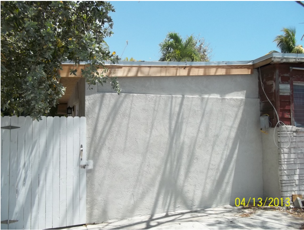
New Door Window and light with a new fence all unpermitted
