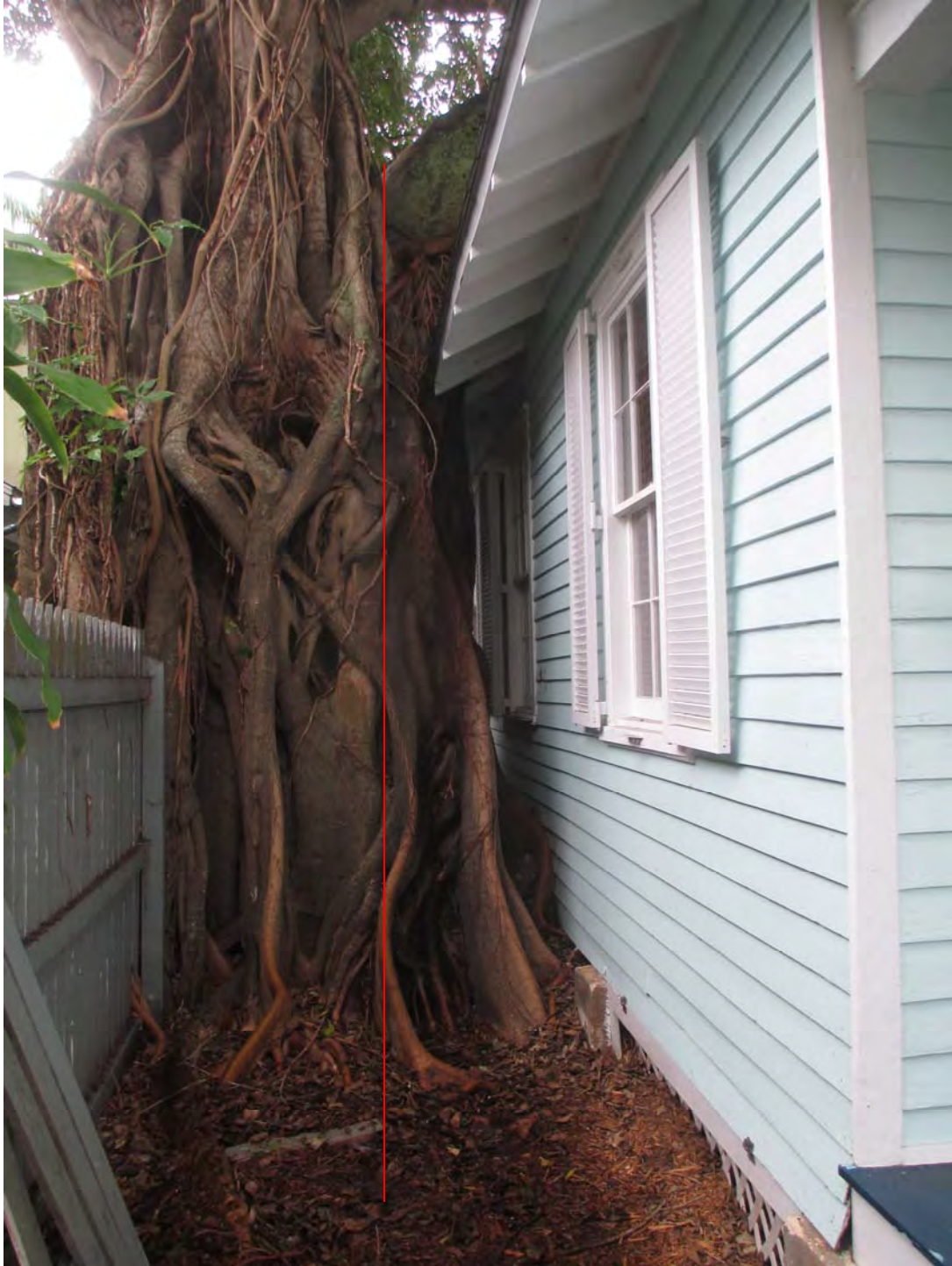
View standing on 818 Carsten Lane. A large section of this tree was able to be removed to prevent the immediate future damage to the house at 818. Note the large amount of roots that appear to be on 820 Carsten Lane, left of the fence. No additional major trimming of this tree can occur at this time.
