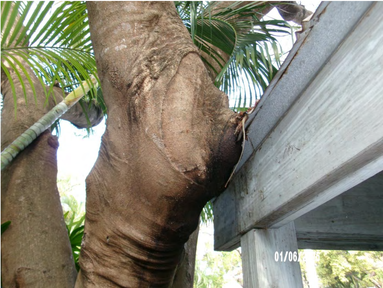
Close up photo of tree trunk against car port roof. Tree is damaged and weeping from impact area.
