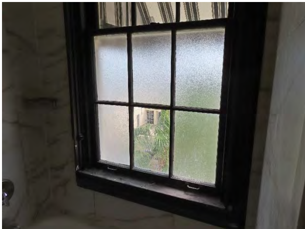
Photo 15: Window located in the shower of room 652 was missing a frosted privacy pane.
