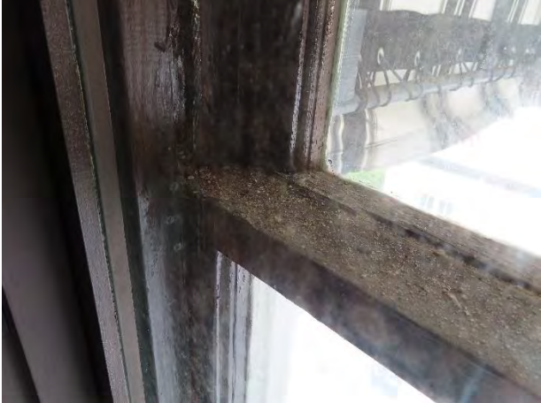
Photo 9: Debris accumulation between the primary window and the interior glazing panes.
