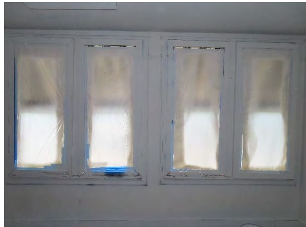
Photo 18: Primary windows missing in room 662. Secondary windows in place with extensive wood decay.
