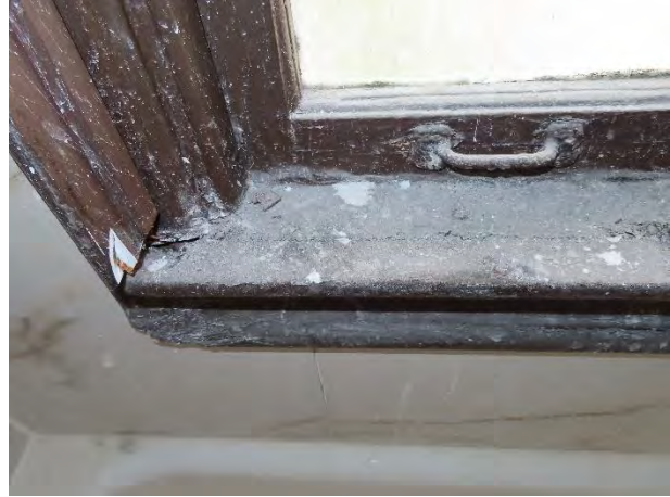
Photo 14: Typical wood rot in the windows located in the showers (photo taken in room 652).
