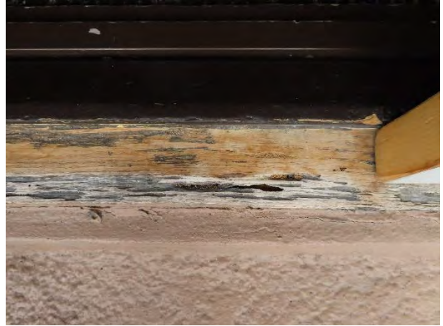
Photo 2: Termite damage at the door sill plate at room 257.
