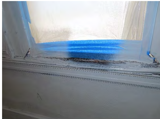
Photo 16: Wood rot from water infiltration in room 662.
