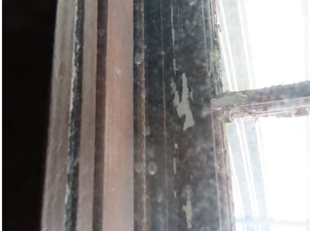
Photo 10: Deteriorated paint was observed at some locations between the primary and secondary assemblies.
