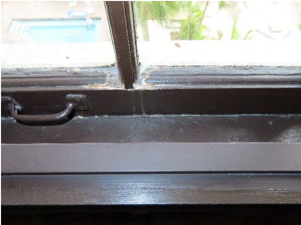
Photo 11: Water staining was observed at most of the windows.
