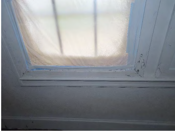
Photo 13: Termite damage to wood frames in room 641.
