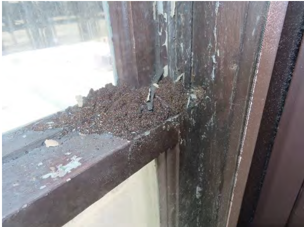
Photo 12: Debris accumulation from termites.
