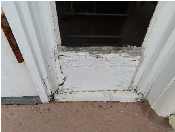
Photo 3: Deterioration caused by water at room 261.
