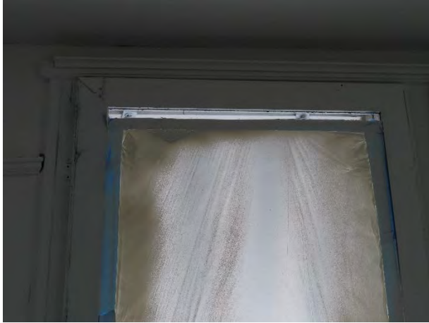
Photo 19: Gaps above the secondary glazing in room 662 at the missing windows allows air and water to enter the building.
