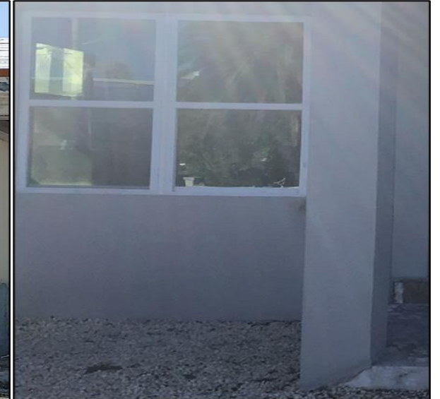
No flood vents 2023
