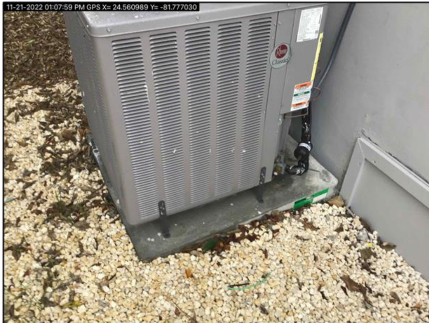
Condenser unit on grade and a covered flood vent
