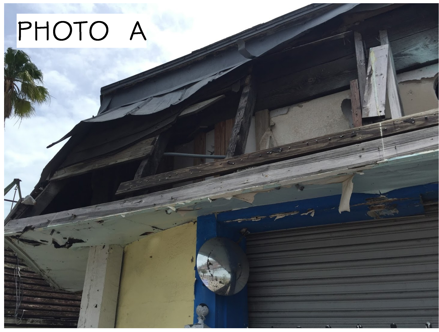
REMOVE EXISTING METAL ROOFING, FRAMING DETERIORATED SOFFIT & DOORS
