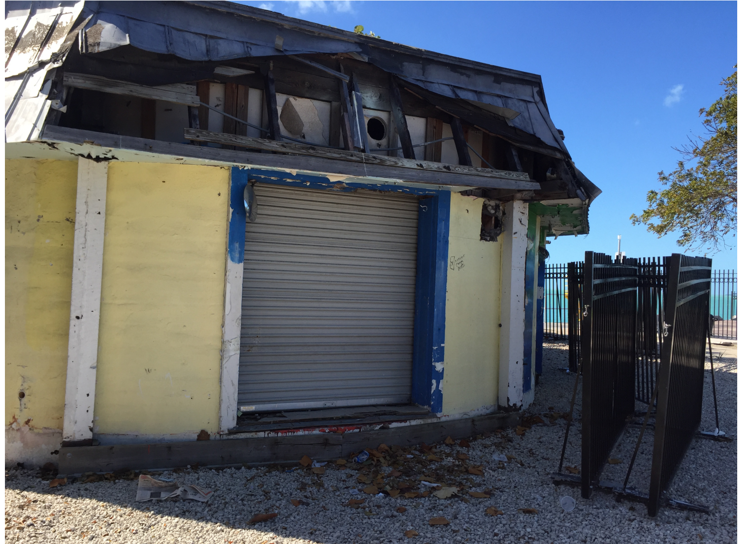
REMOVE ALL EXISTING DOORS AND ROOFING. ALL HISTORIC TIMBERS COLUMNS & BEAMS TO REMAIN AND REPAIRED AS REQUIRED
