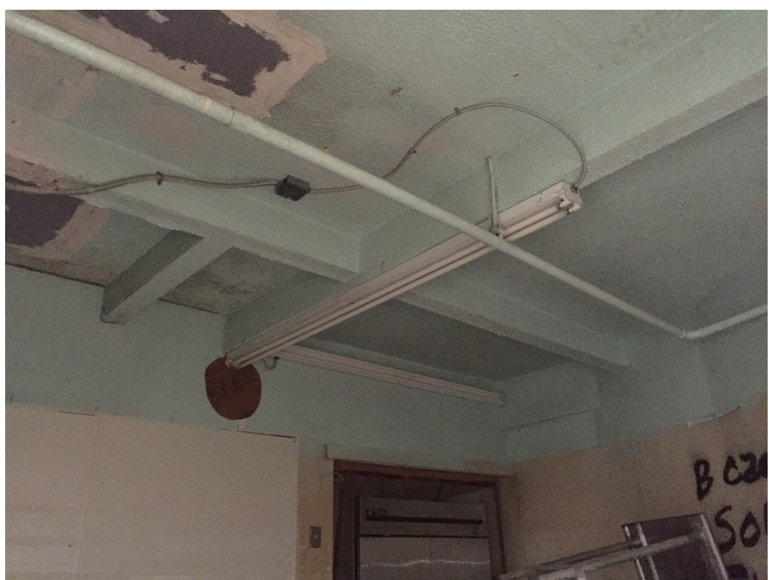
EXISTING CABLE HUT INTERIOR REMOVE ALL INTERIOR NON HISTORIC MATERIALS AT WALLS AND ROOF
