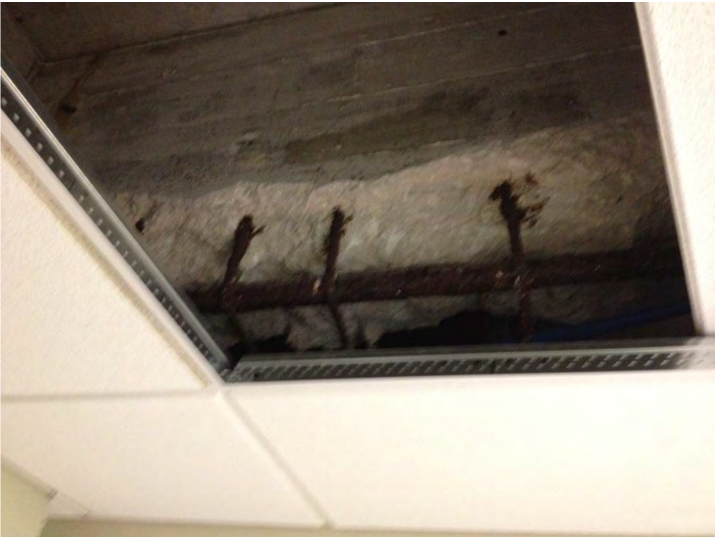
Note missing 6" plus of concrete with exposed severely rusted rebar
