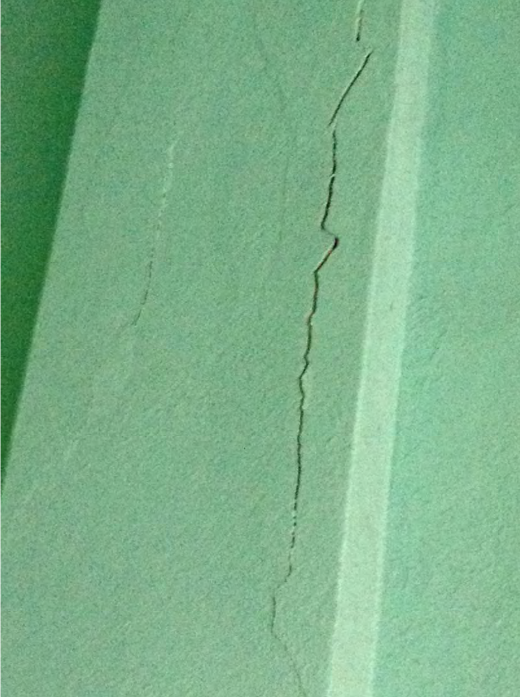
Note cracking along steel reinforcing
