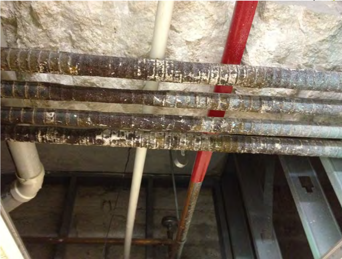
Note bottom of concrete beam has been chipped away
