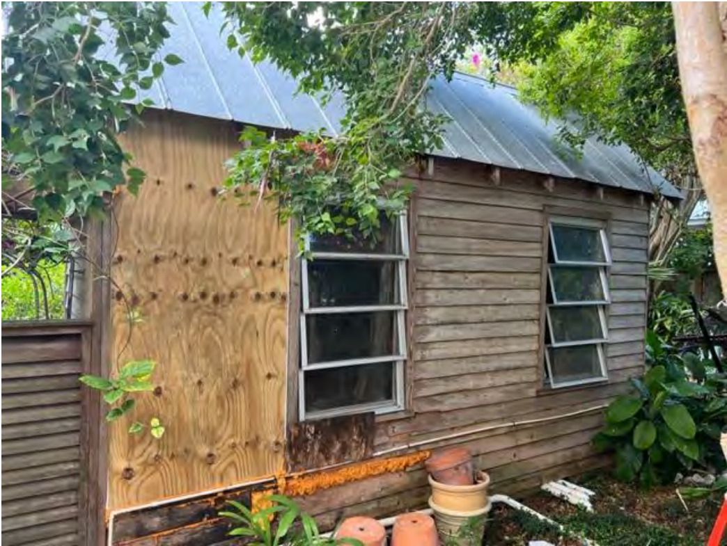
219 Olivia Shed, built in 2000. Rear (east) elevation. Extensive bee damage.
