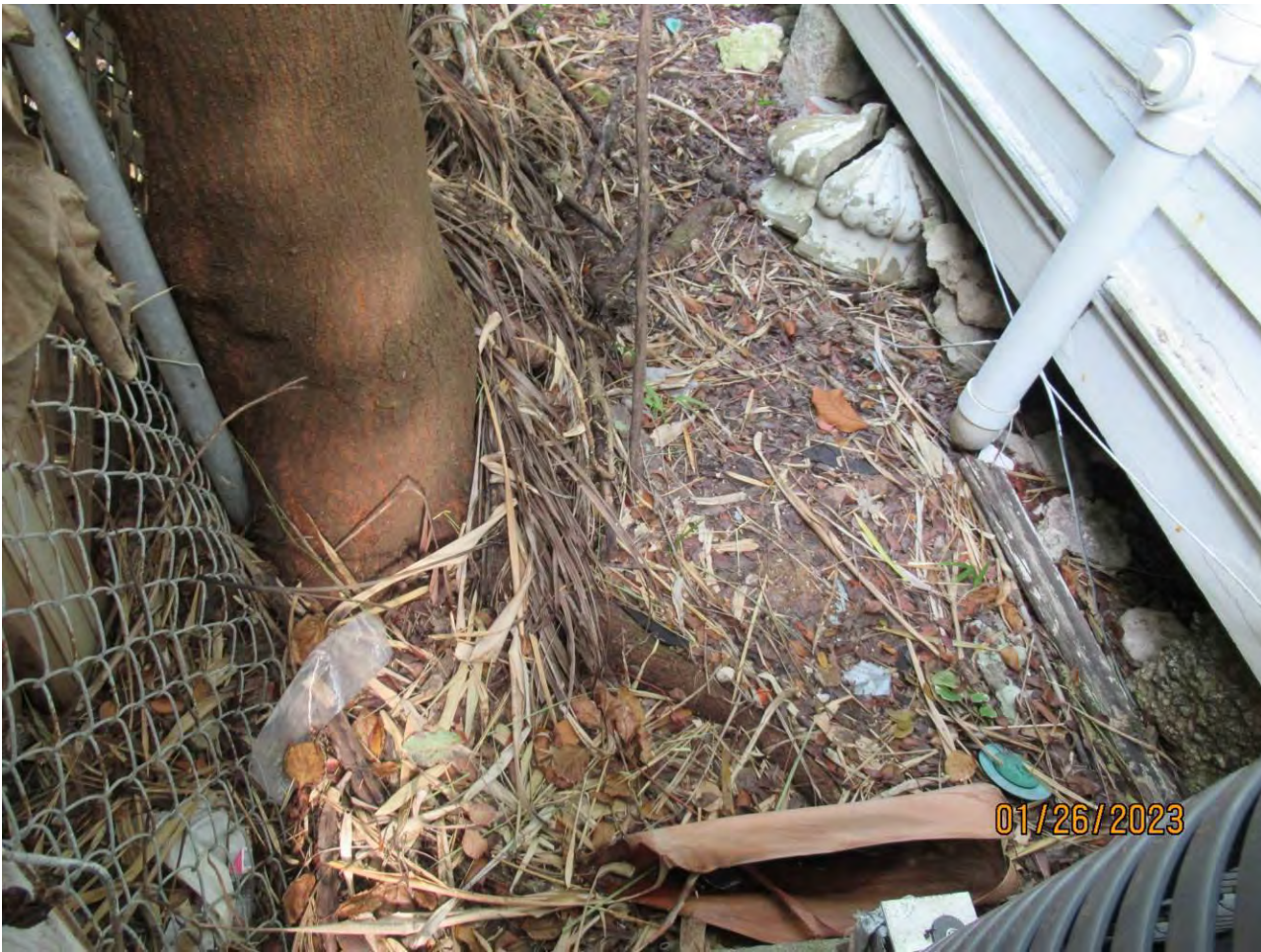
Photo of base of tree in relation to structure (829 Eaton). Fence on left is the property line.
