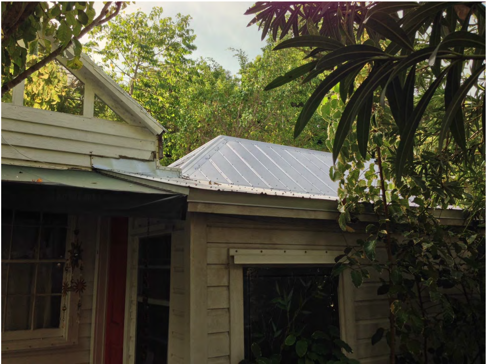
Roof that is hip in the front and gable in the rear. The V-Crimp roof is more recent.
