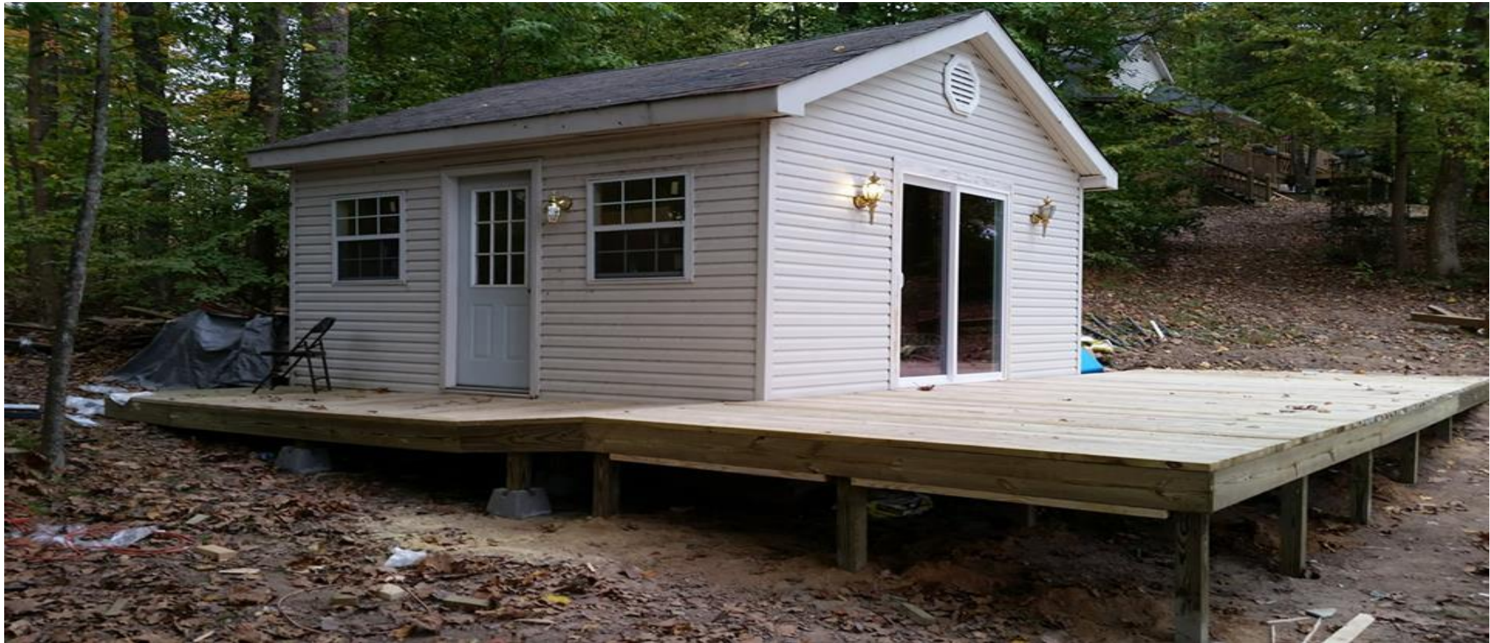
FOUNDATION BAD DESIGN AND CONSTRUCTION
