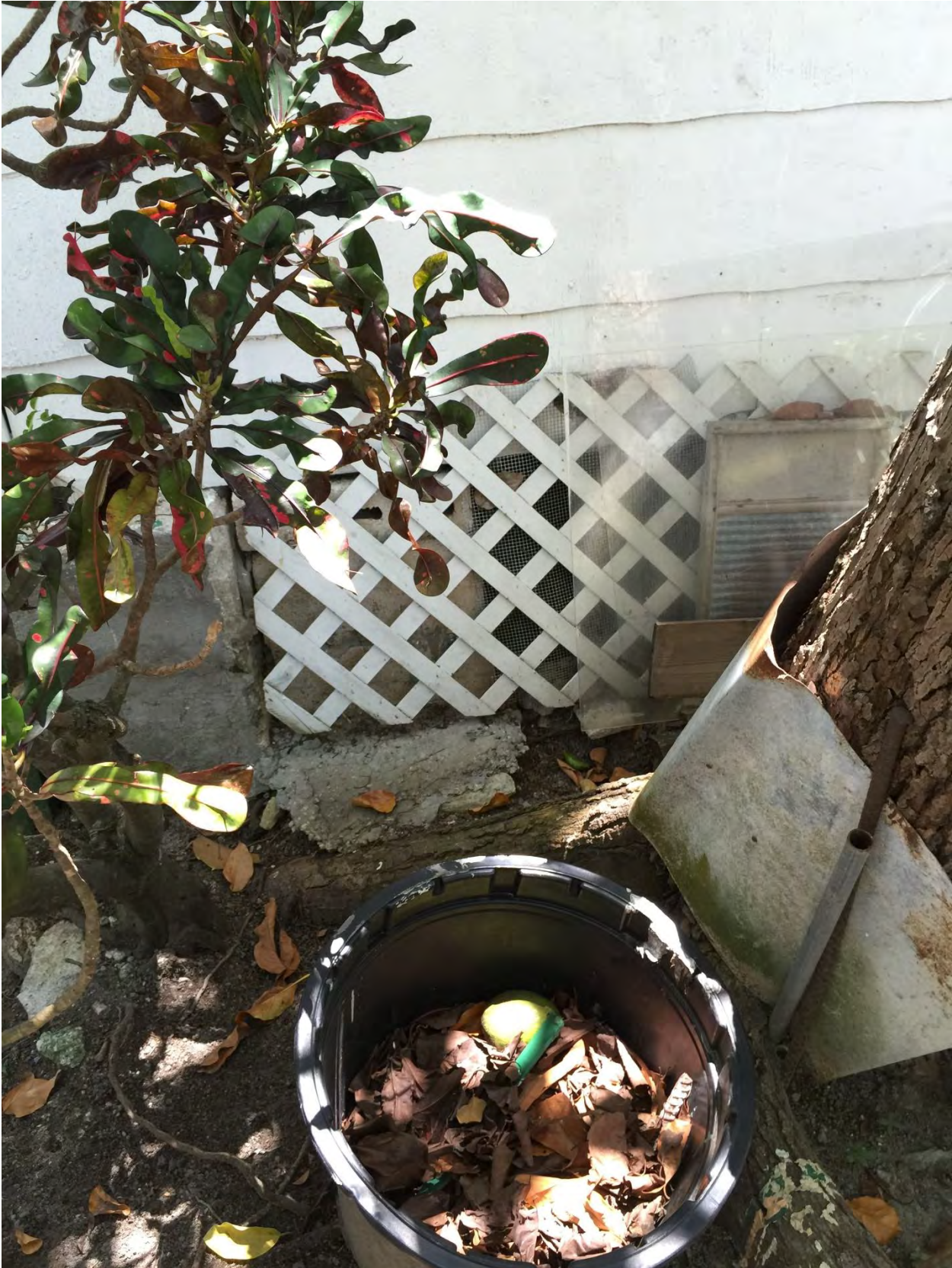
Roots intruding on foundation
