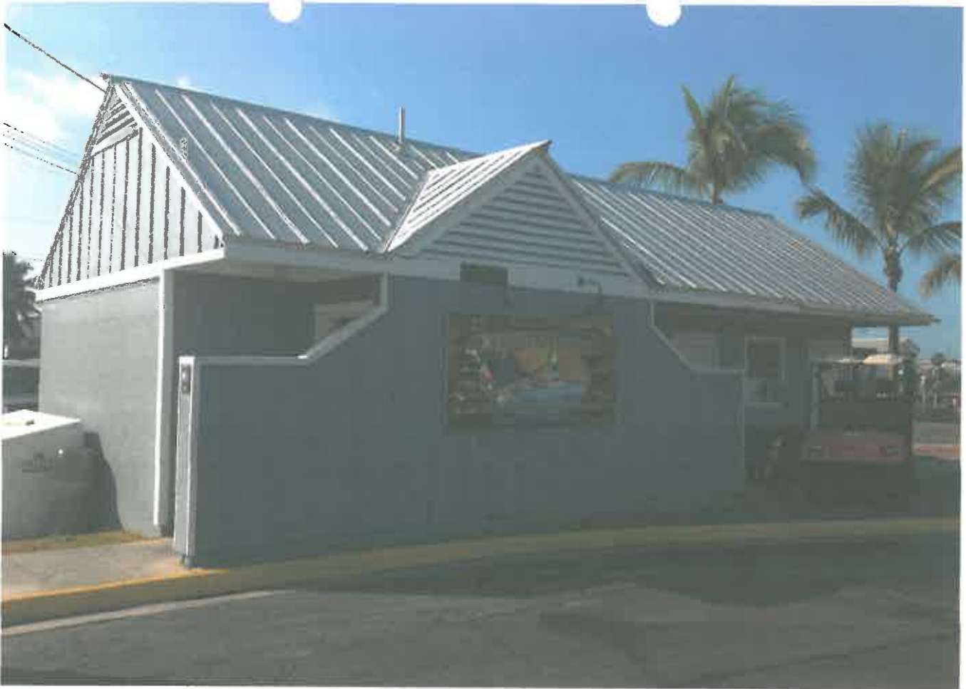
RESTROOM BUILDING TO BE REPLACED
