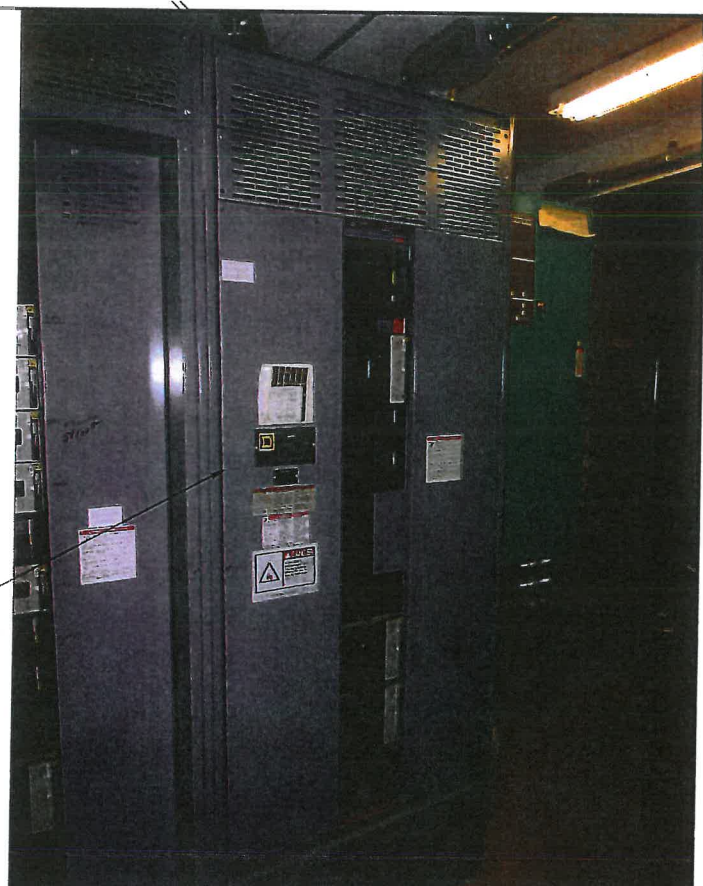
2ND FLOOR MAIN ELECTRICAL ROOM SWITCHGEAR
