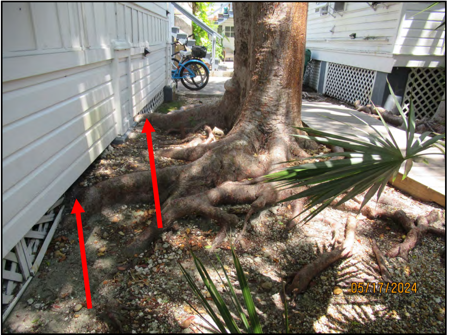
Root system of gumbo limbo #1, impeding crawl space of structure to the left.
