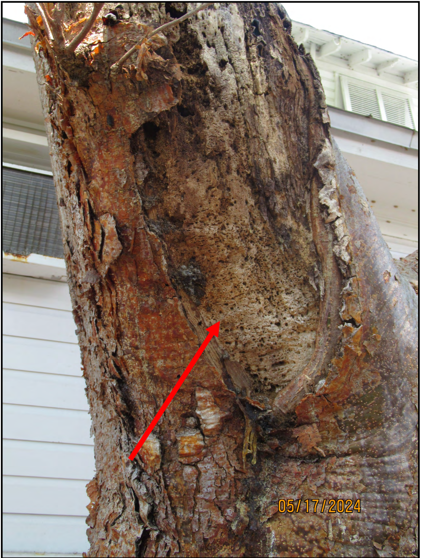
GL1: Closer view of borer and termite damage
