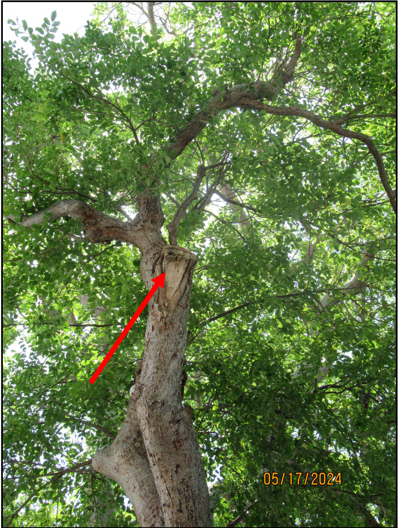
GL1: Large limb improperly pruned resulting in torn and ripped down the trunk
