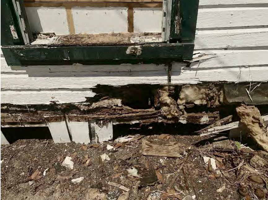
DETERIORATED FRONT SILL BEAM AT SIDE ADDITION
