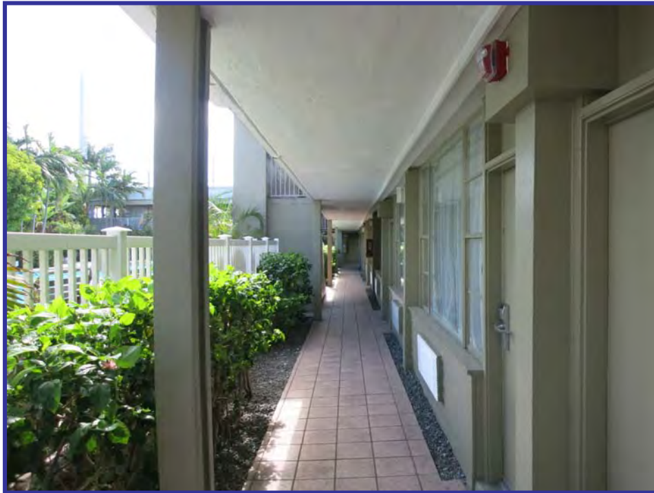
View looking south along the east elevation of the 2-story north building (ground floor)
