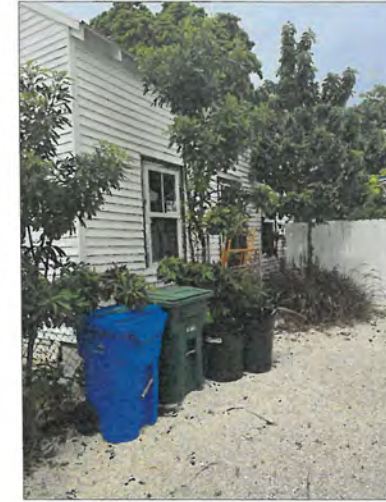
5 RIGHT SIDE VIEW A0.2 LOOKING FRONT TO BACK, REPLACE EXISTING WITH IMPACT 2 OVER 2 WINDOWS
