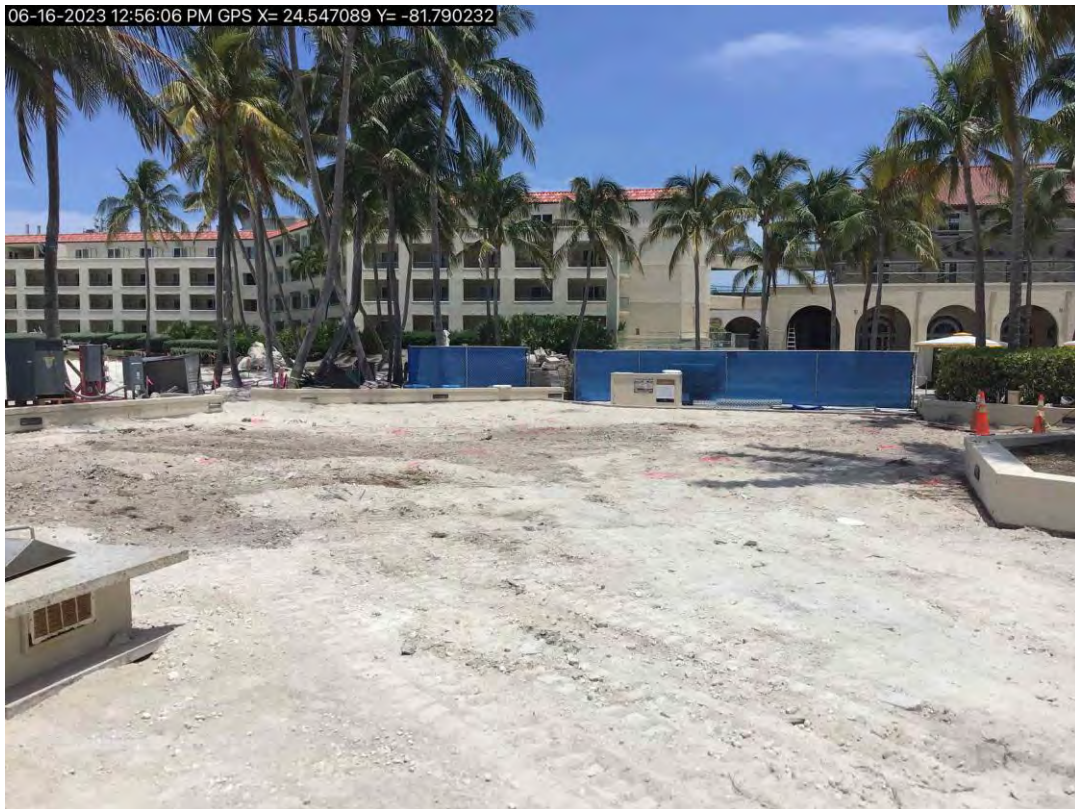
Photo depicting where the west structure used to be. Photo from TrakIt file BLD2023-0135 as part of the inspection for demolition.
