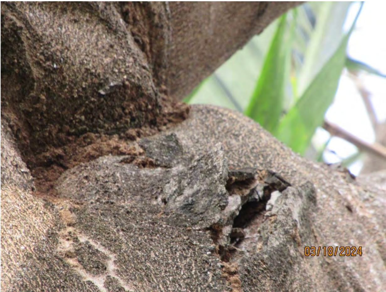
Two close up photos of canopy/trunk connection area showing termites trails.
