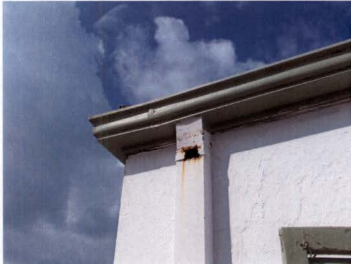
Detail of damaged gutters and downspouts at main house. Gutters and downspouts will be replaced with new copper units matching the historic profile. All of the gutters are piped into the historic cistern located under the Florida Room of the house.
