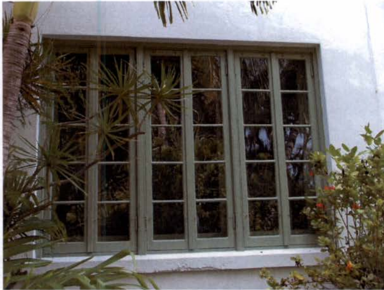
Typical first floor casement window. The windows are termite damaged, and will be replaced with new mahogany impact-resistant casement windows. Profiles will match exactly.
