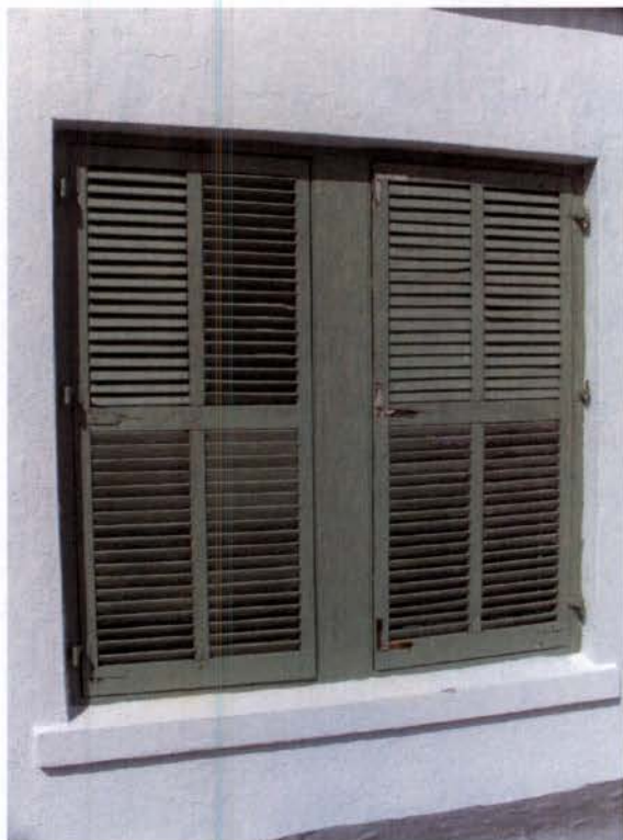
Typical second floor window (shuttered). Both windows and shutters have structural damage from termites.
