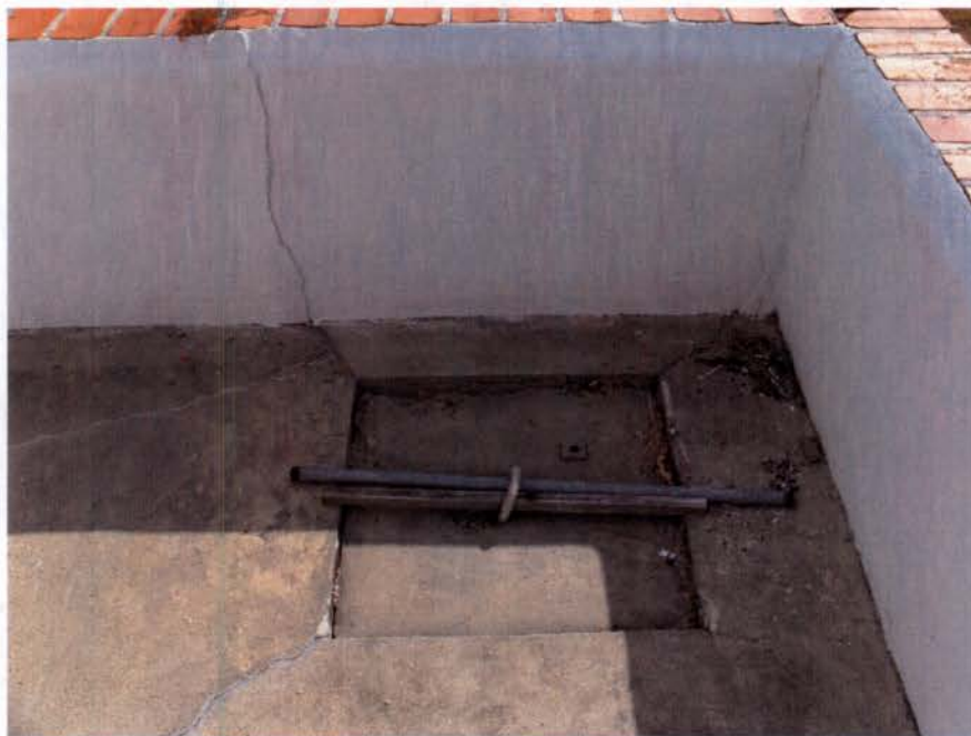
The cover to the historic cistern is located on the porch. The cistern is functional, and will remain so.
