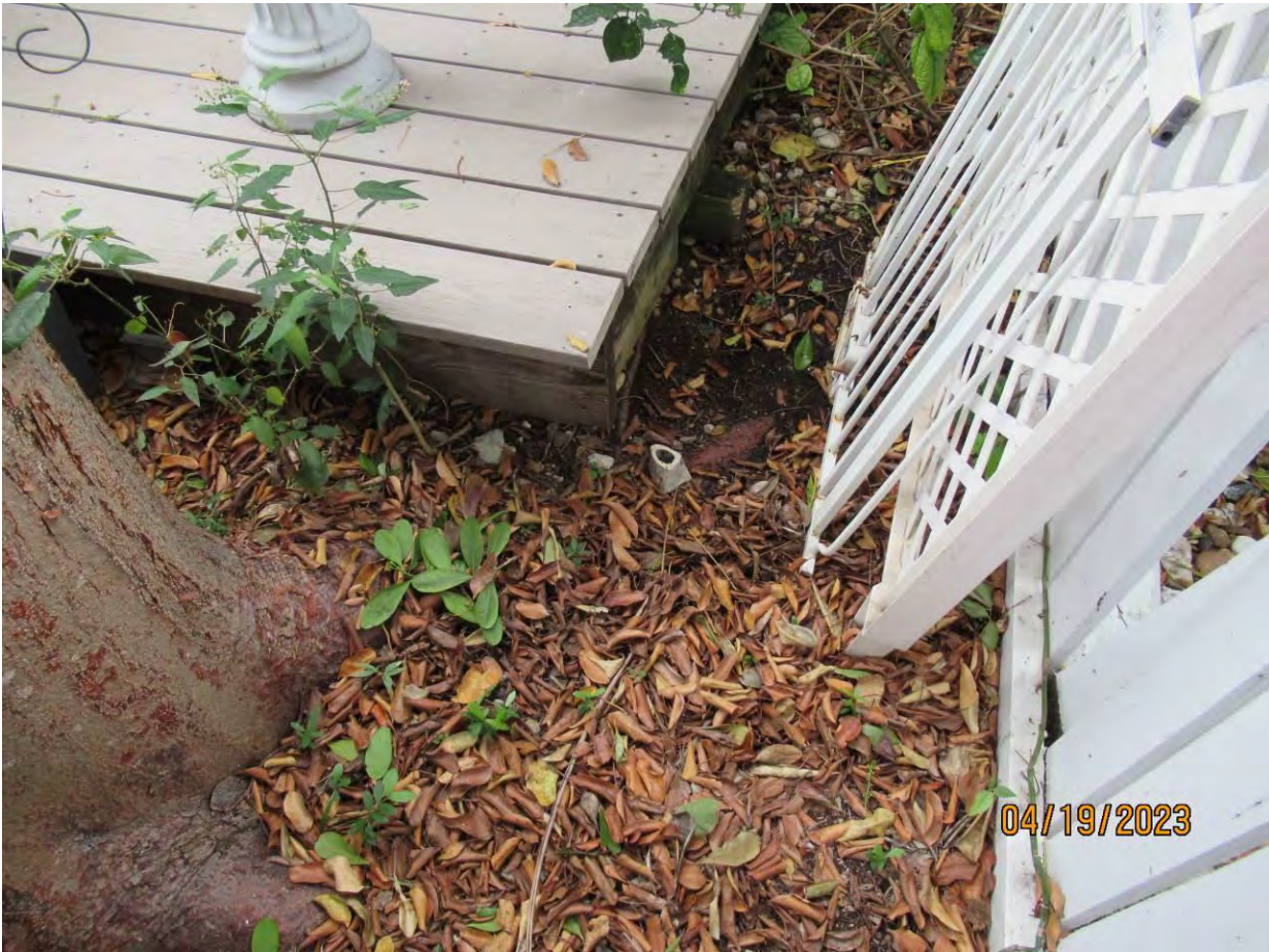
Photo of base of tree and deck, view 1.
