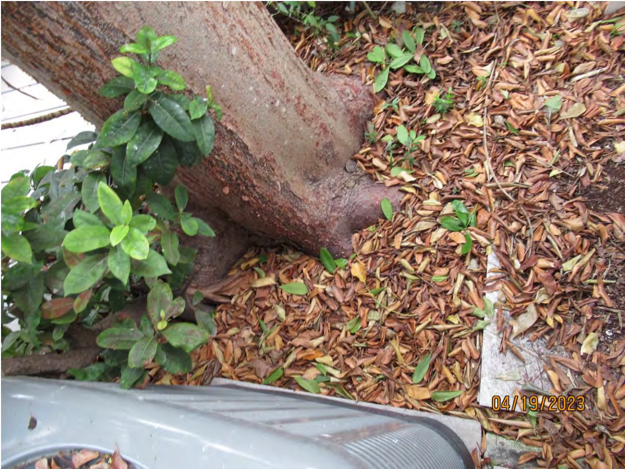
Two photos of base of tree and its roots in relation to ac unit.
