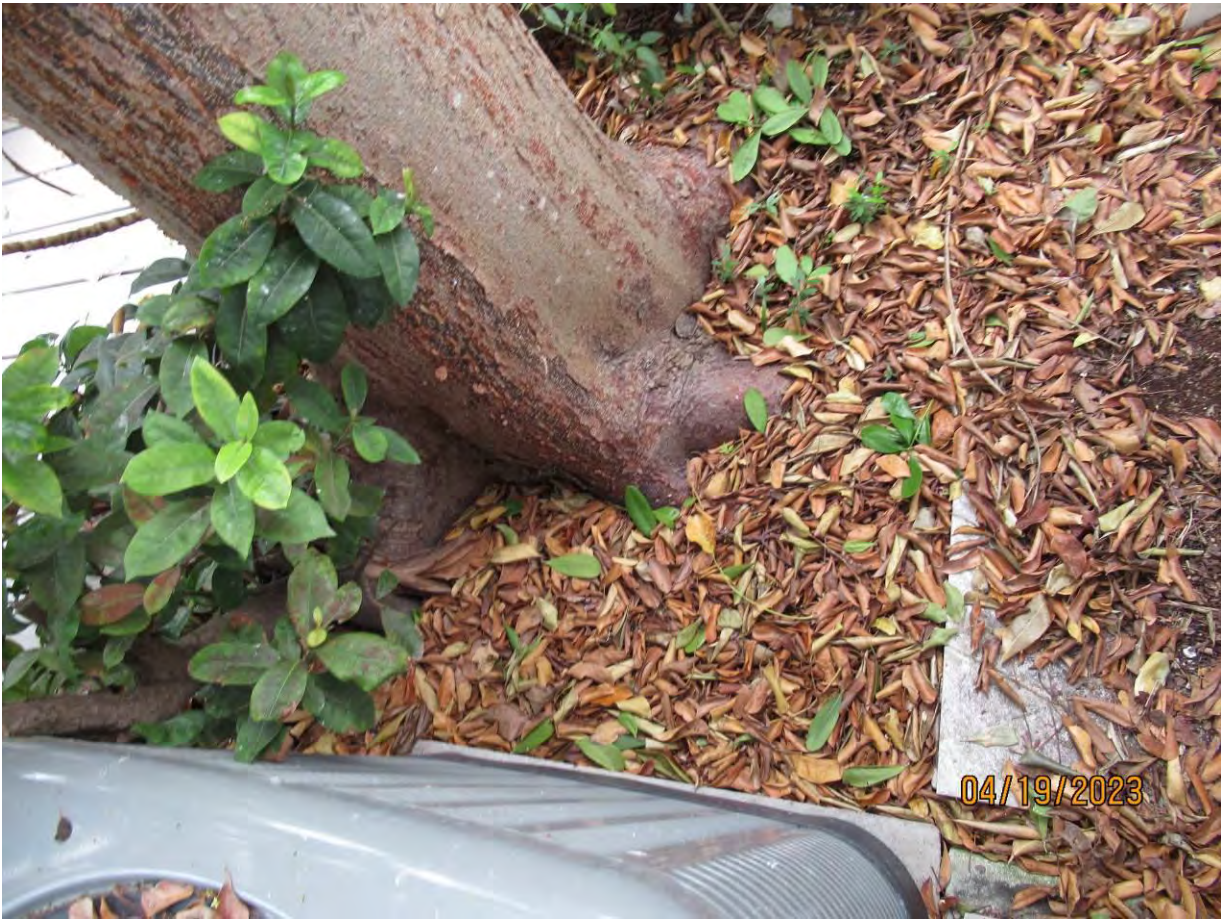
Two photos of base of tree and its roots in relation to ac unit.
