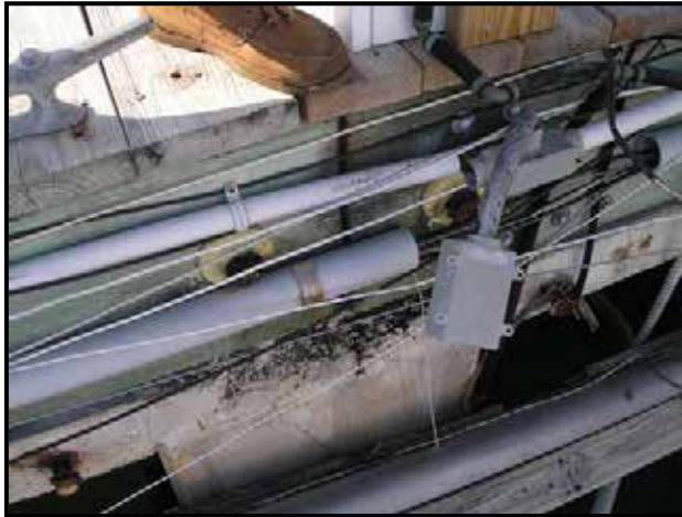
Photo of wood deck and wood substructure resting on concrete deck supported by concrete pilings encased on a concrete cap.
