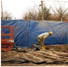
Preparing to excavate tar well after placing sheet piling around a structure.
