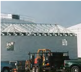
For Tampa Bay Water, Black & Veatch designed a new building to house an aqua ammonia storage/feed system and process water booster pump station. The building was constructed of split-face concrete block with a decorative standing seam metal roof.
