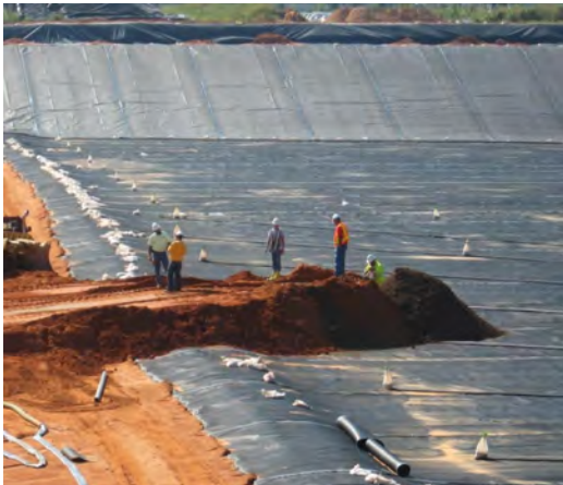
Placing first load of contaminated soil into containment cell constructed at the Escambia Treating Company site.
