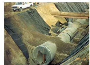
Our diverse sanitary and storm sewer pipeline experience will benefit the Utilities Department when designing or rehabilitating piping systems of any size and material, including ductile iron, PVC, steel, and HDPE.
