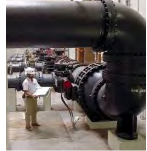
The Utilities Department will benefit from Black & Veatch's experience and expertise in virtually every type of pumping condition, pumping equipment, piping size and material, control scheme and power source.
