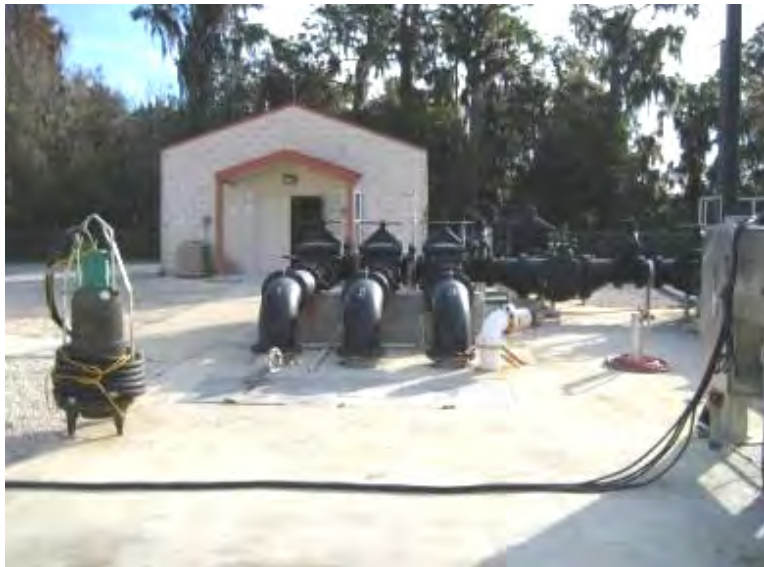
The facilities were designed to be neighborhood friendly taking into consideration odor, noise, and aesthetics.
