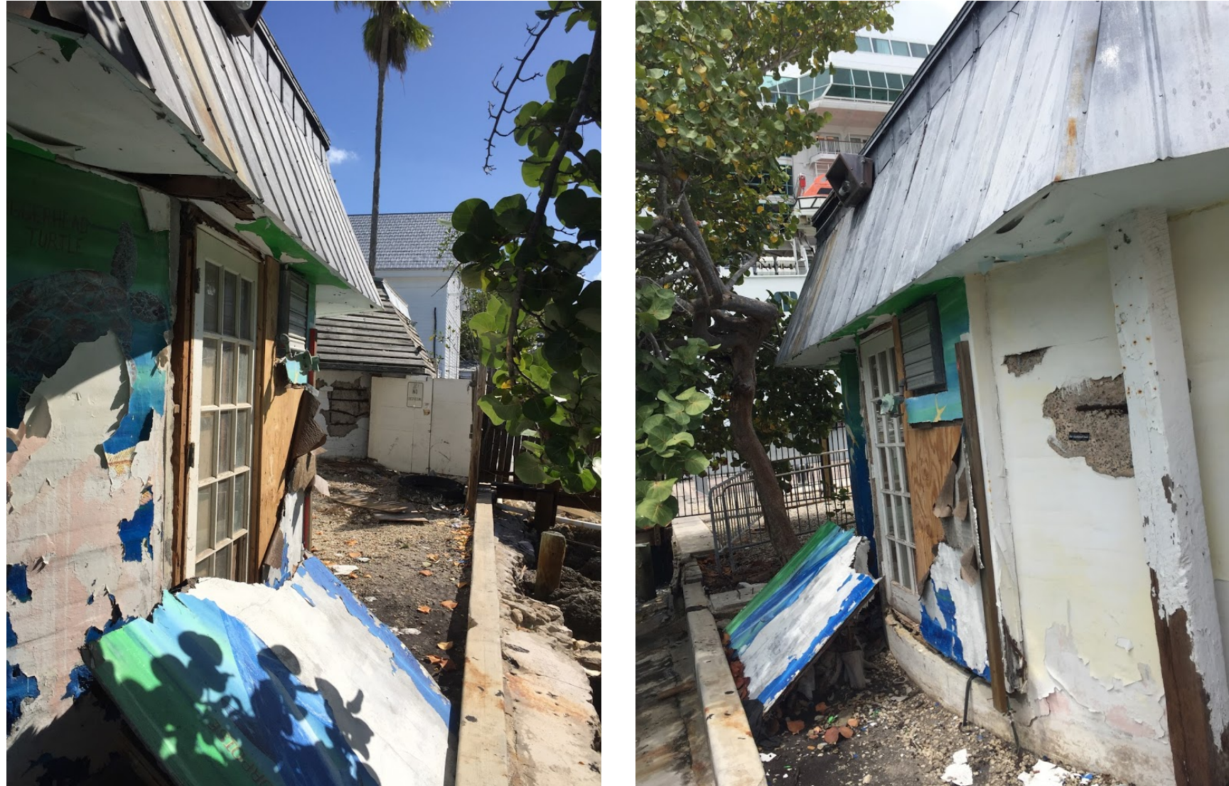
REMOVE ALL EXISTING DOORS AND ROOFING. REPAIR ALL CONCRETE SPALLING AT WALLS
