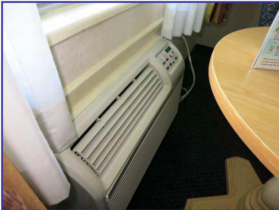
Typical air-conditioning unit
