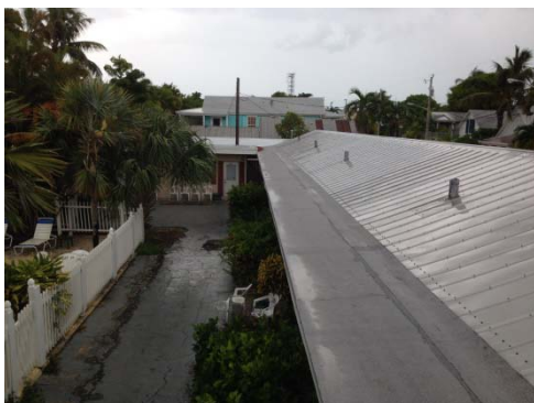
Photograph 6 showing inadequate fire separation between the L shaped building on the left and the adjacent structure. Note the non-code compliant egress windows.
