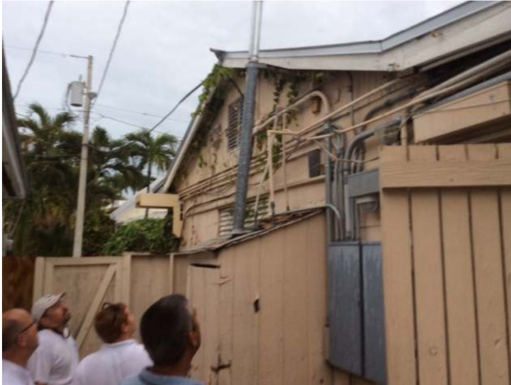
Rear structure addition and roof. Electrical systems are out of code.
