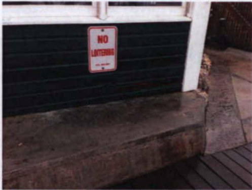
(Pic. 1) Exterior cladding (Deterioration from moisture)
