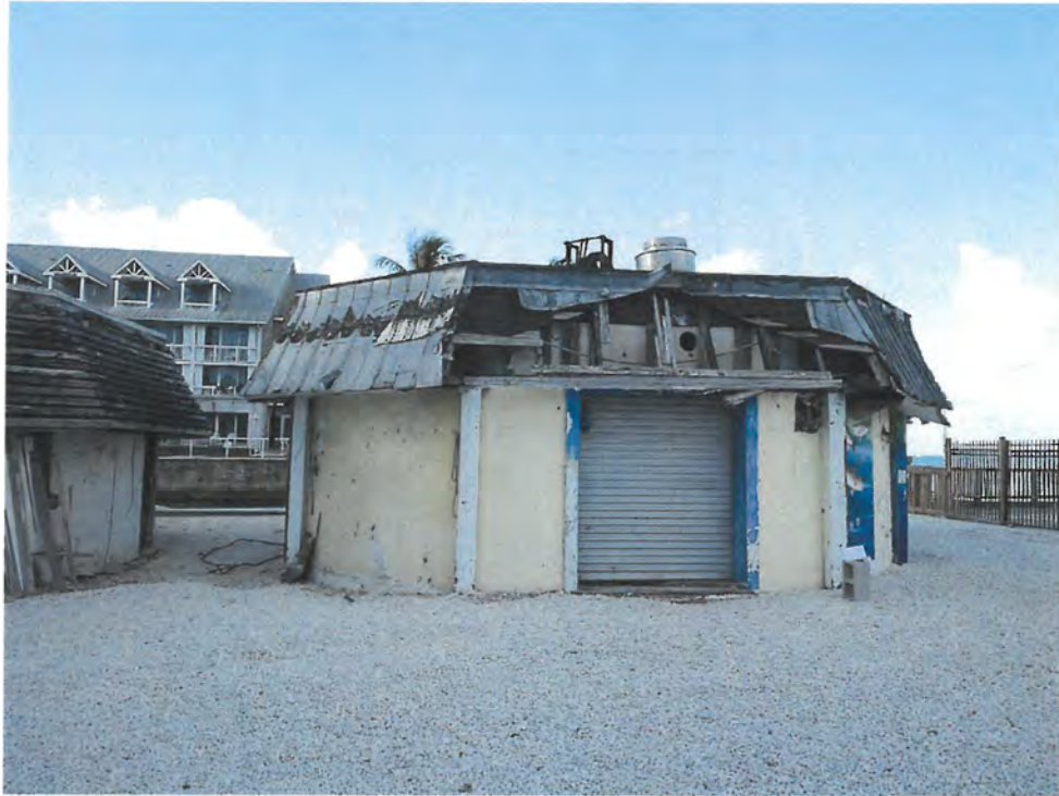
West Cable Hut showing metal mansard roof that is to be replaced with matching horizontal slat roof to match the East Cable Hut.
