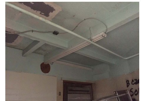
EXISTING CABLE HUT INTERIOR REMOVE ALL INTERIOR NON HISTORIC MATERIALS AT WALLS AND ROOF
