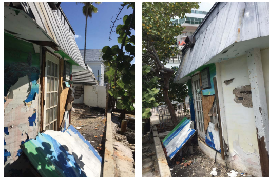
REMOVE ALL EXISTING DOORS AND ROOFING. REPAIR ALL CONCRETE SPALLING AT WALLS
