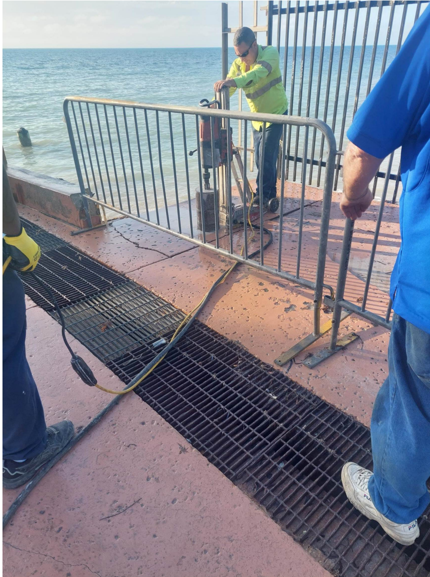
Location 4. Existing condition of concrete sidewalk. Coring by City of Key West Community Services.
