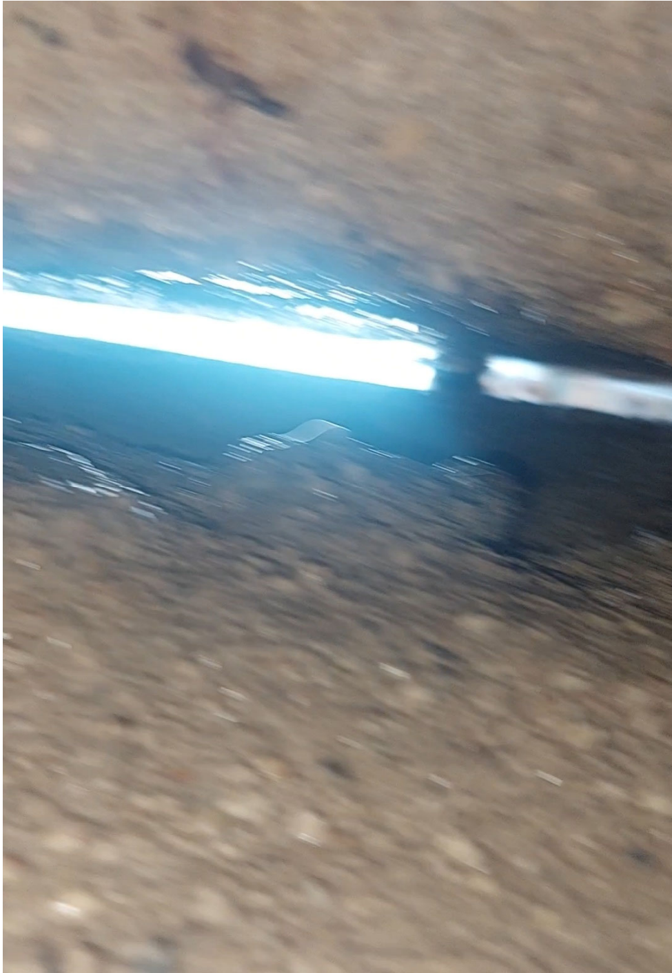
Location 4. Existing condition of concrete sidewalk. Open void below the sidewalk slab. Gap toward the open water.
