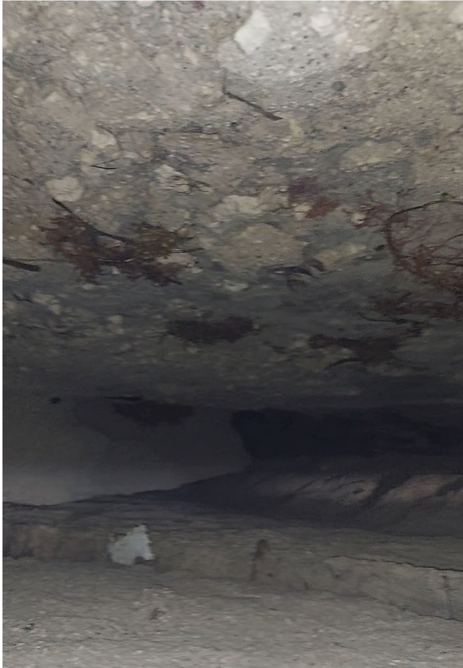
Location 4. Existing condition of concrete sidewalk. Open void below the sidewalk slab.
