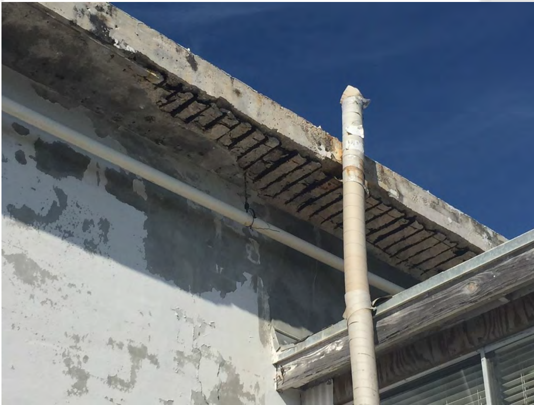
FRONT FAÇADE - EXISTING ROOF CONDITION WITH SPALLING DAMAGE
