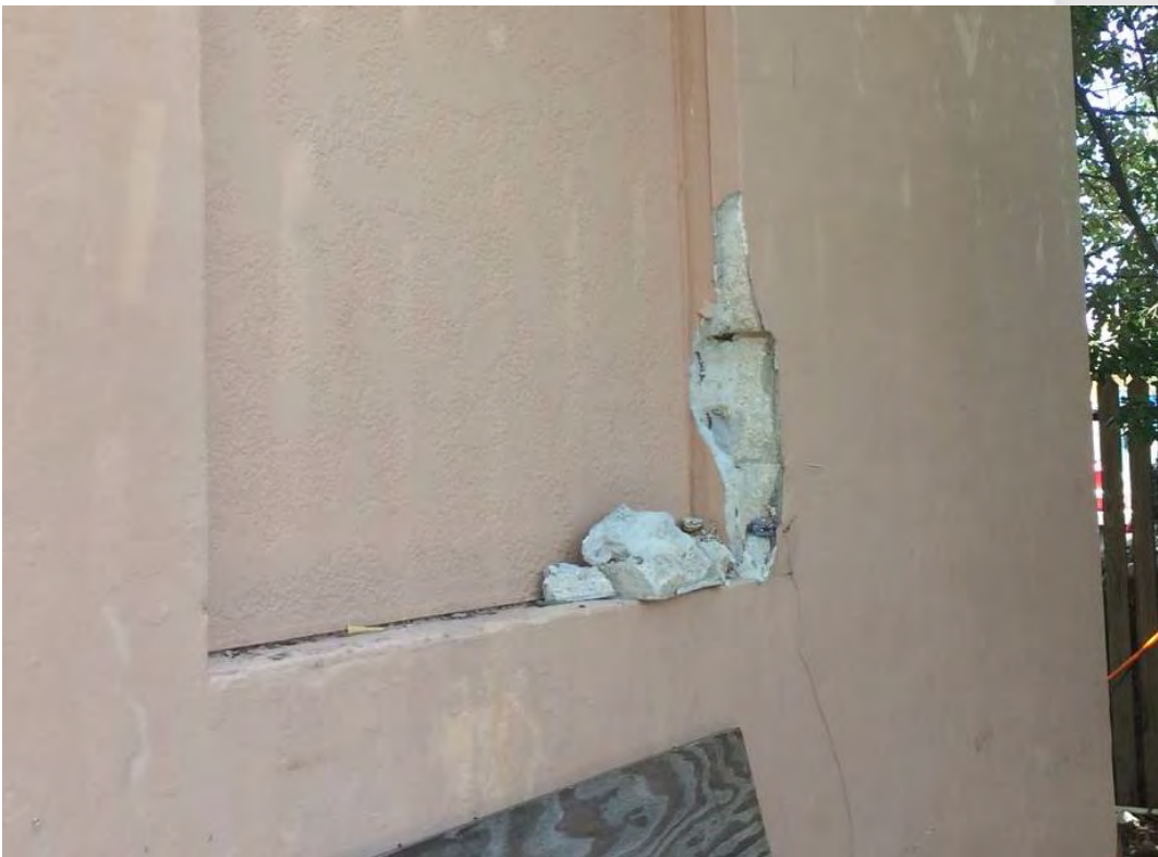
SPALLING DAMAGE AT EXISTING REAR FACADE
