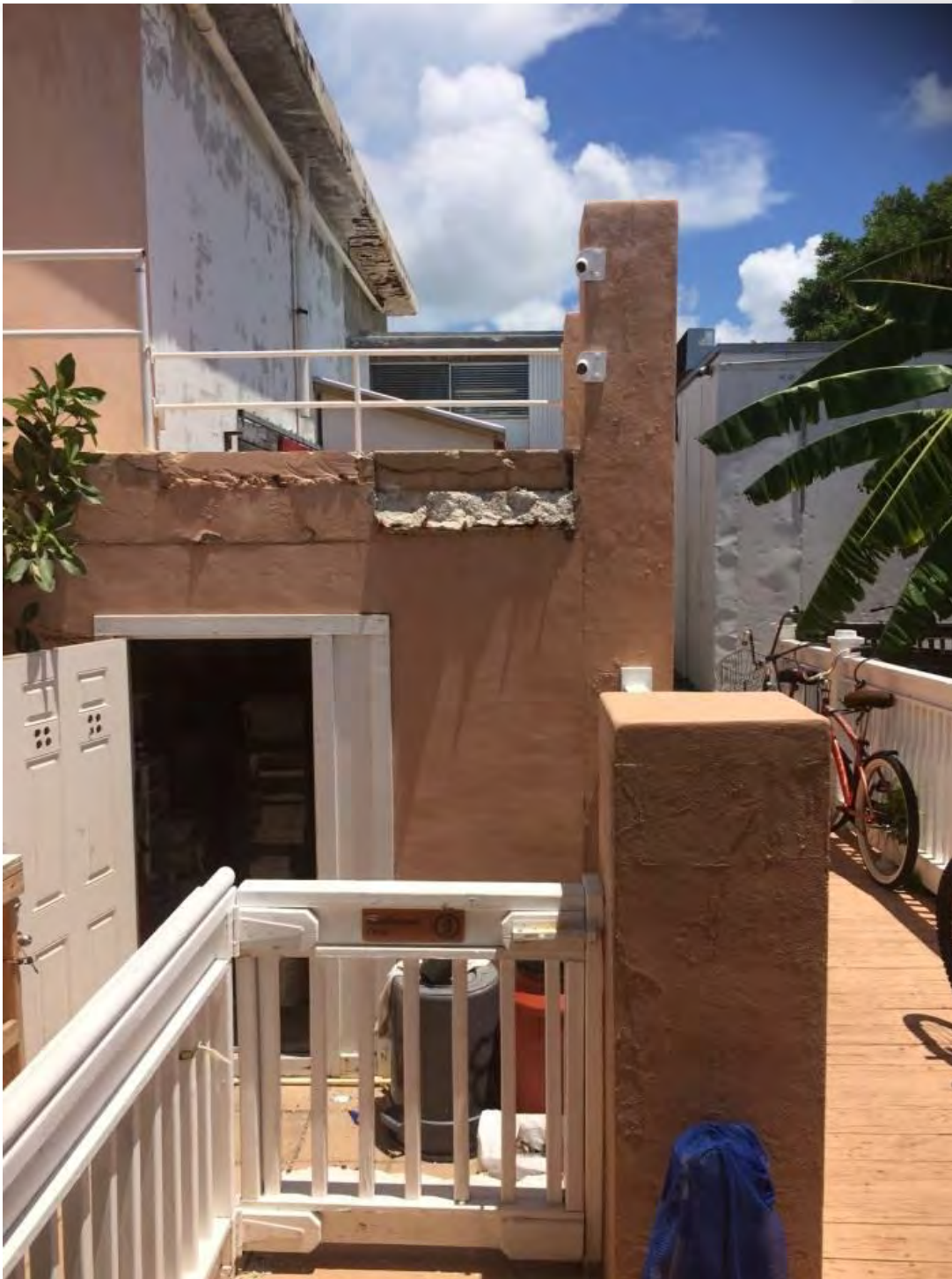
EXISTING CONDITION WITH SPALLING DAMAGE
