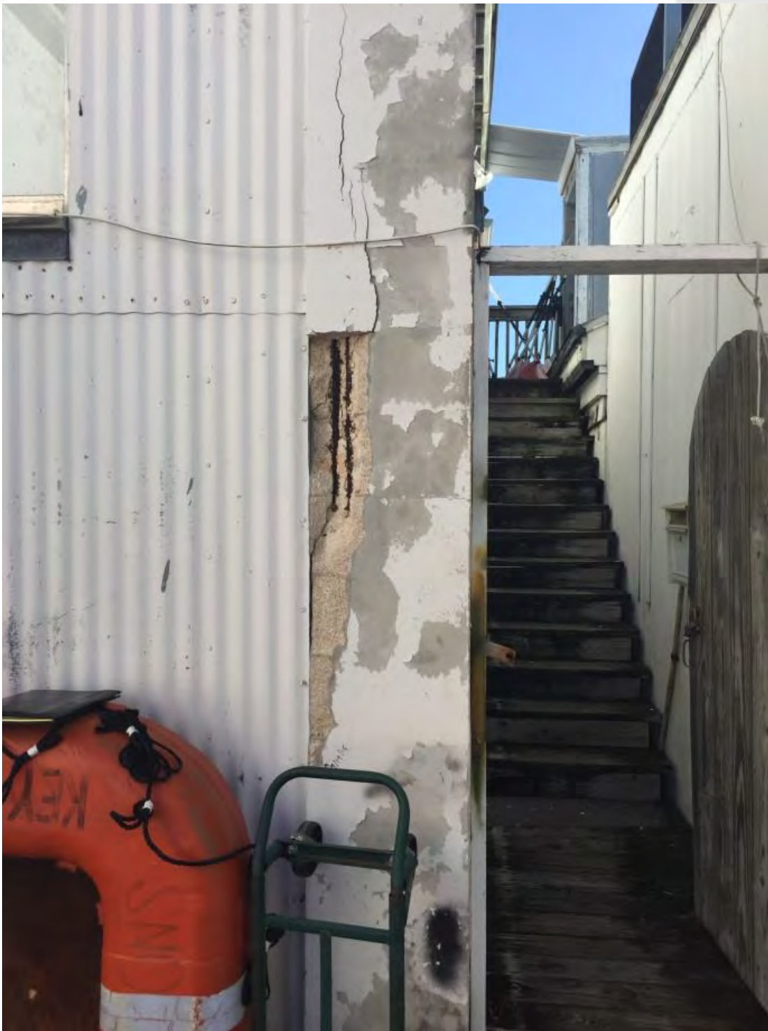
SPALLING DAMAGE AT EXISTING CONCRETE COLUMN
