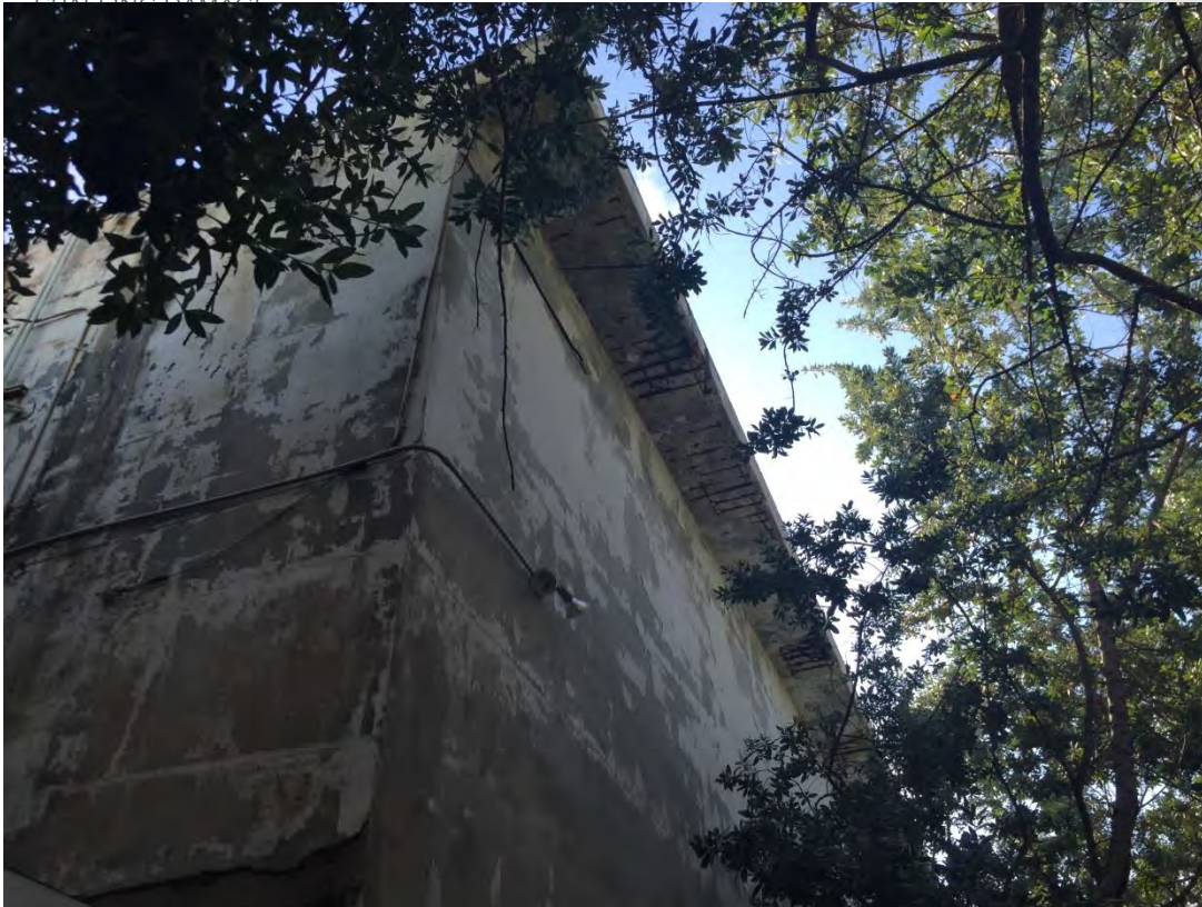
REAR FAÇADE - EXISTING ROOF CONDITION WITH SPALLING DAMAGE
