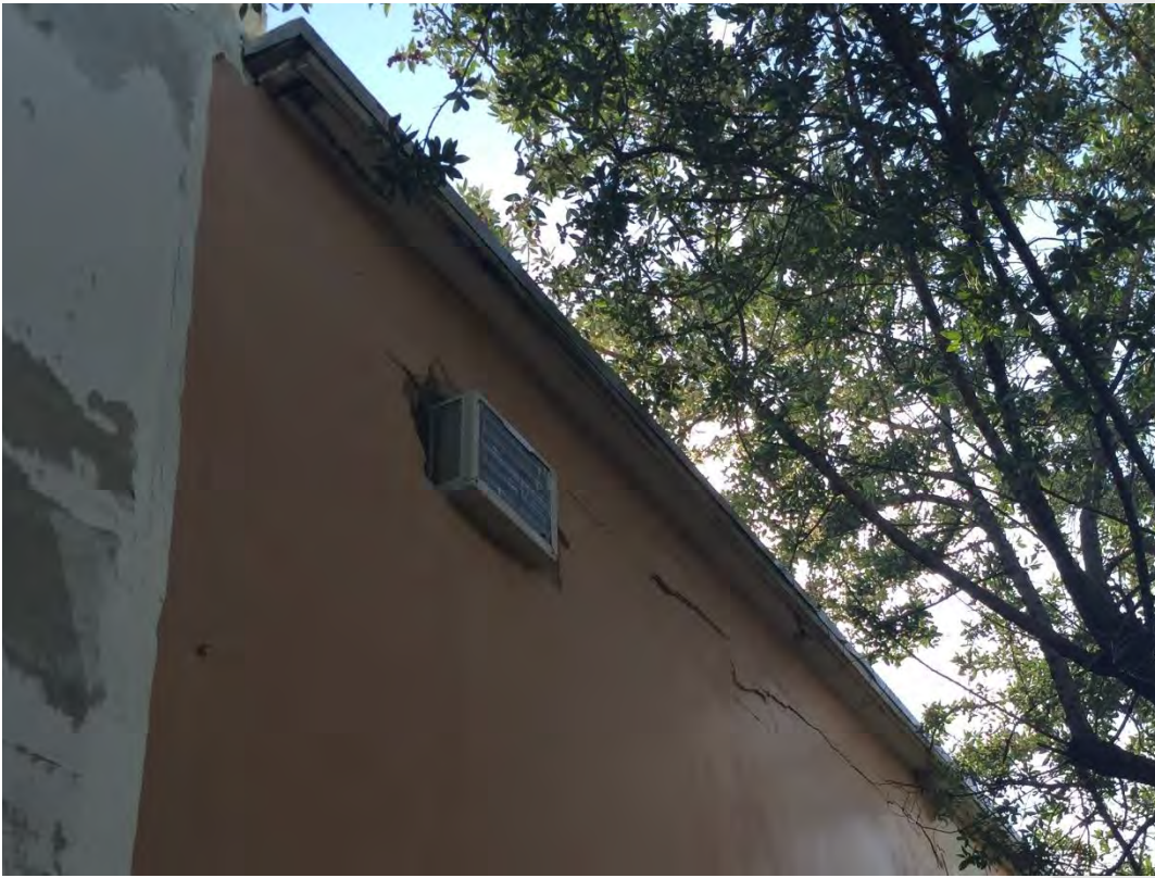
SPALLING DAMAGE AT EXISTING REAR FACADE
