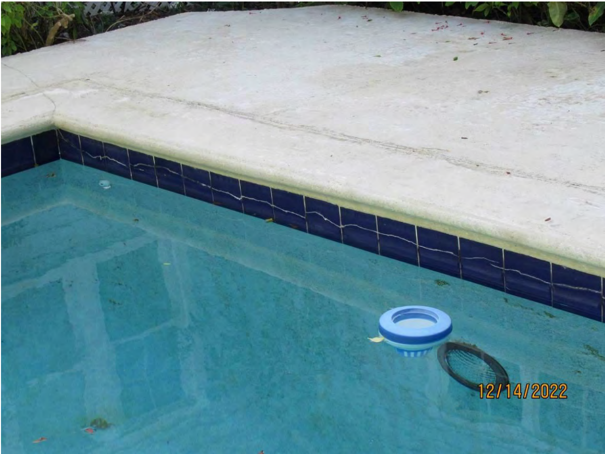
Photo of crack in pool tile closest to house.
