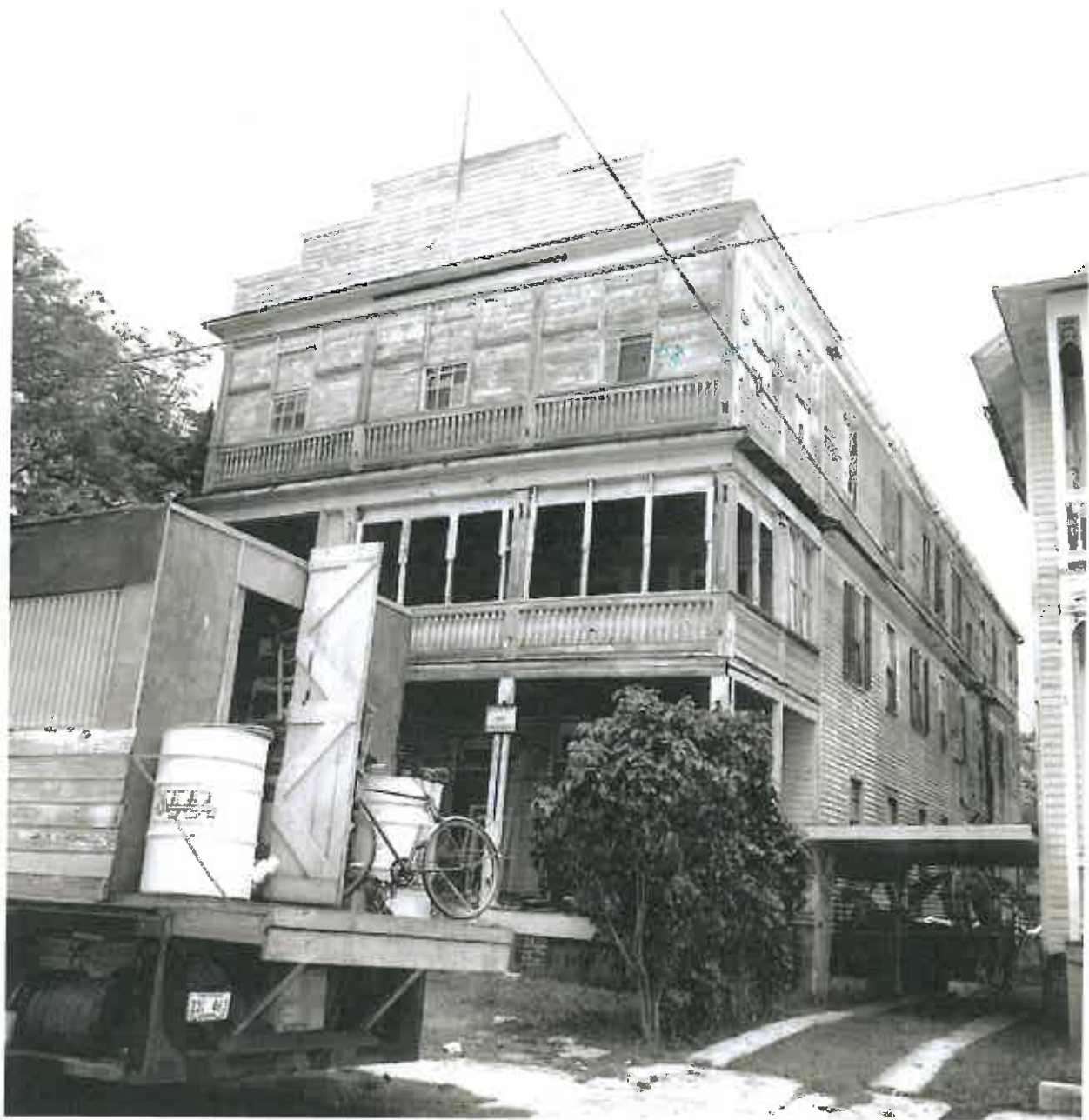
Hotel at 411 William Street before it was restored in 1978. From the Monroe County Library Collection
