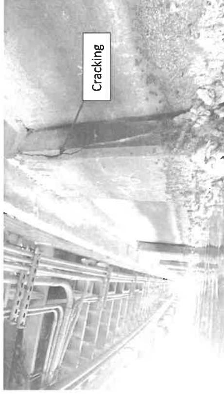
Deficiency B-75: Pile 114 (Station 8+27)
