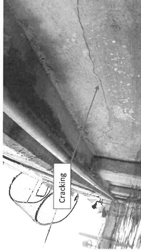
Deficiency A-14: Panel 18-19 (Station 1+50)
