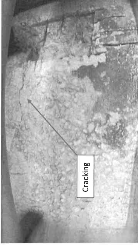
Deficiency A-1: Panel 3-4 (Station 0+14)
