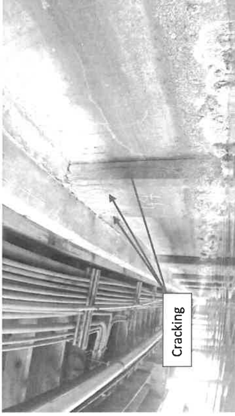
Deficiency B-56: Pile 89 (Station 6+27)
