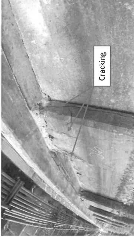
Deficiency B-47: Pile 68 (Station 4+63)
