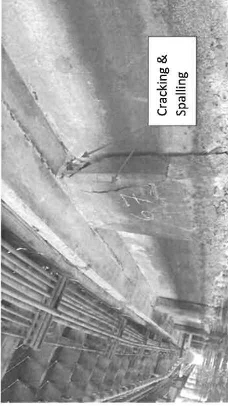
Deficiency B-71: Pile 109 (Station 7+88)
