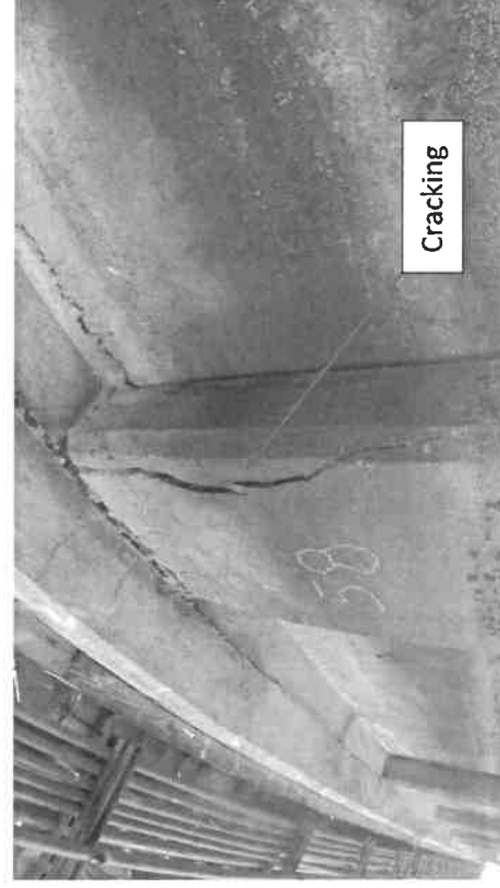
Deficiency B-62: Pile 100 (Station 7+15)
