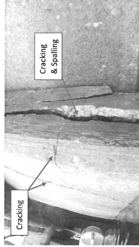
Deficiency A-15: Pile 21 (Station 1+67)
