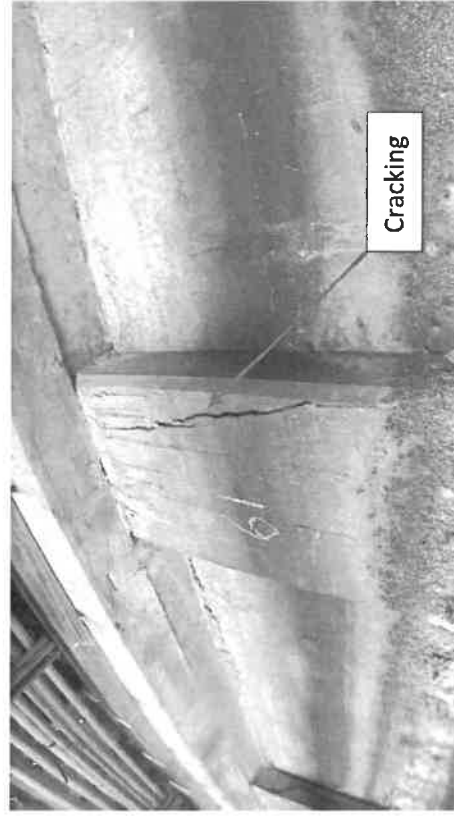
Deficiency B-65: Pile 103 (Station 7+38)_1 of 2
