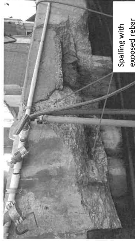
Deficiency A-4: Pile 7 (Station 0+39)
