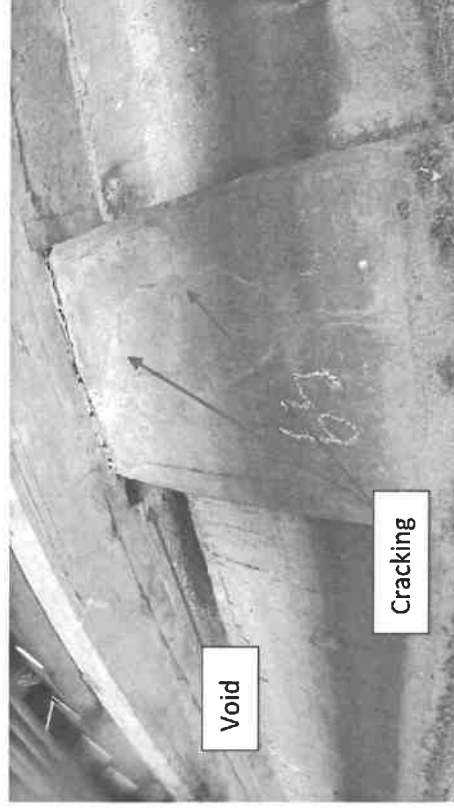
Deficiency B-69: Pile/Cap 107 (Station 7+71)
