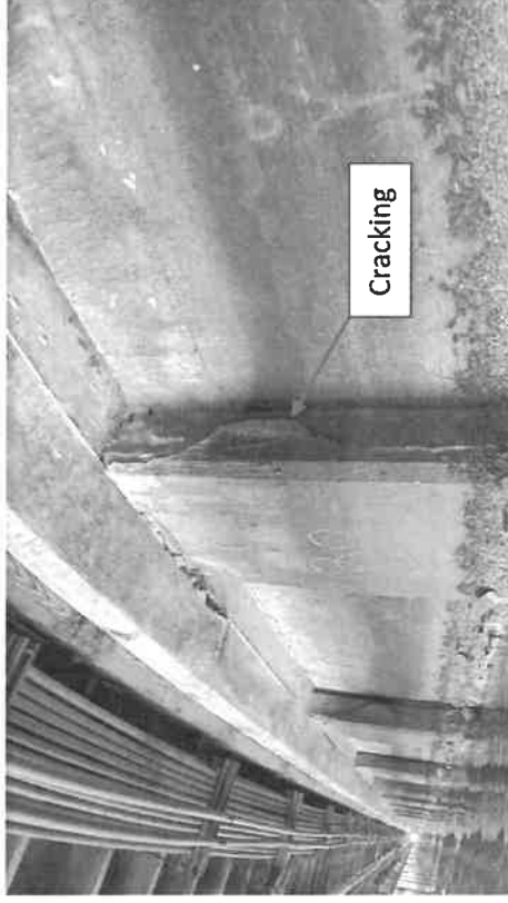
Deficiency B-42: Pile 62 (Station 4+25)
