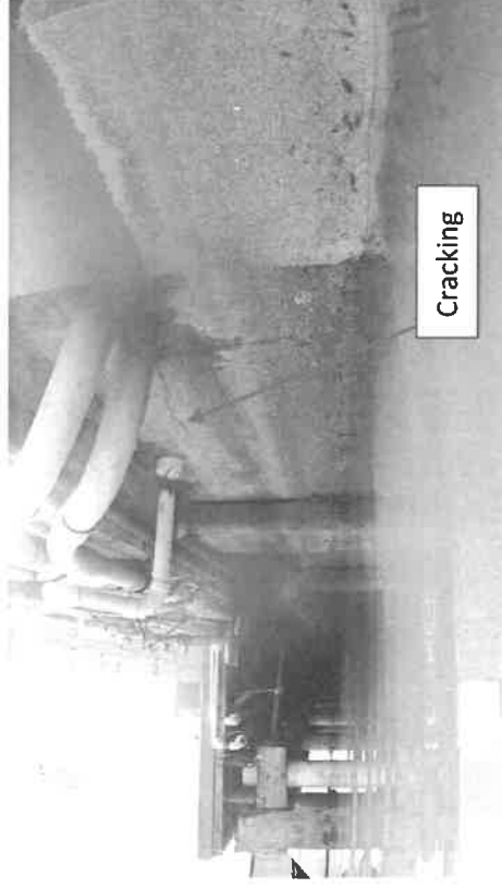
Deficiency B-27: Panel 41-42 (Station 2+93)
