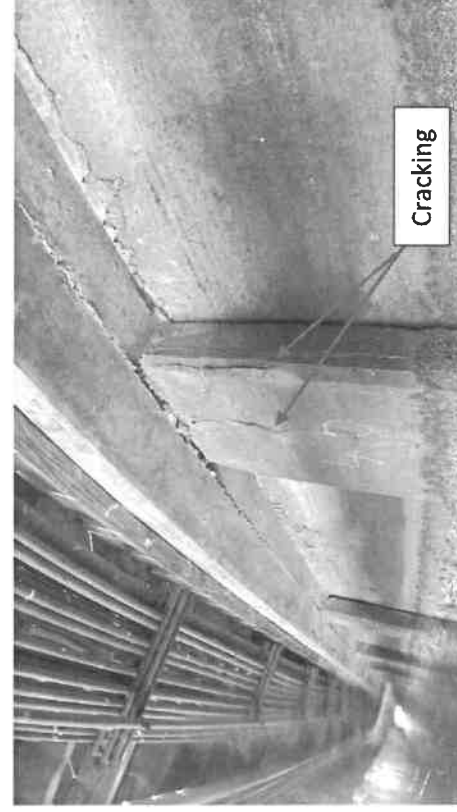
Deficiency B-54: Pile 82 (Station 5+70)
