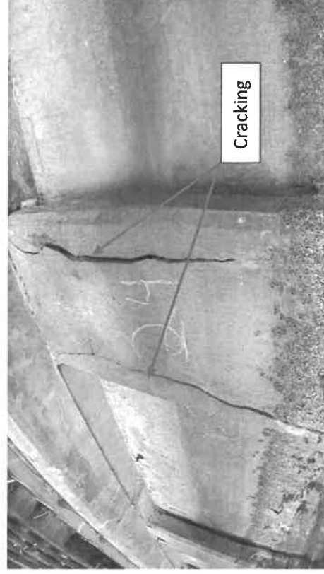
Deficiency B-46: Pile 66 (Station 4+50)
