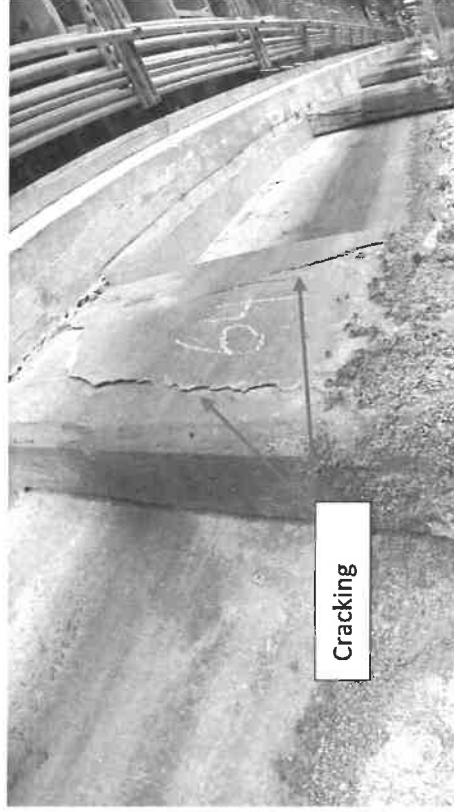
Deficiency B-68: Pile 106 (Station 7+63)
