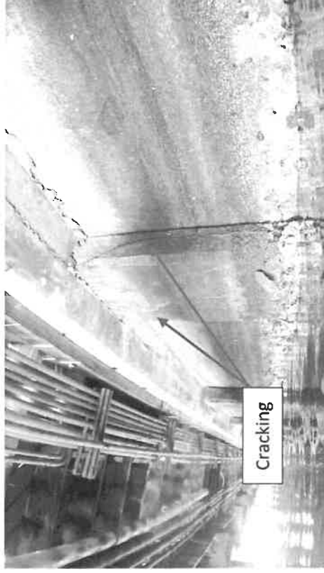
Deficiency B-60: Pile 97 (Station 6+90)
