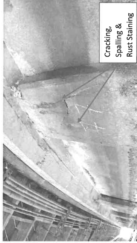
Deficiency B-80: Pile 119 (Station 8+67)
