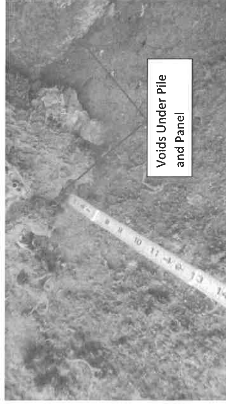
Deficiency B-72: Panels 111-116 (Station 8+03 to 8+38)
