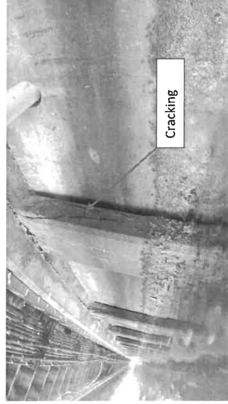
Deficiency B-40: Pile 59 (Station 4+05)
