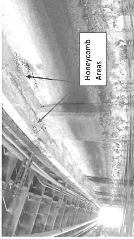
Deficiency B-83: Cap @124-127 (Station 9+04 to 9+25)_1 of 2
