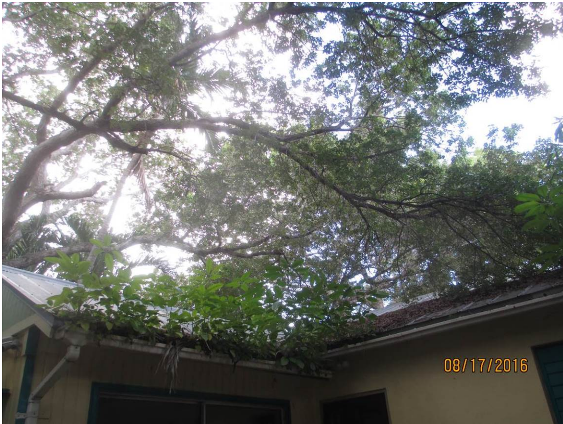
Photos above show canopy branches growing over existing structure
